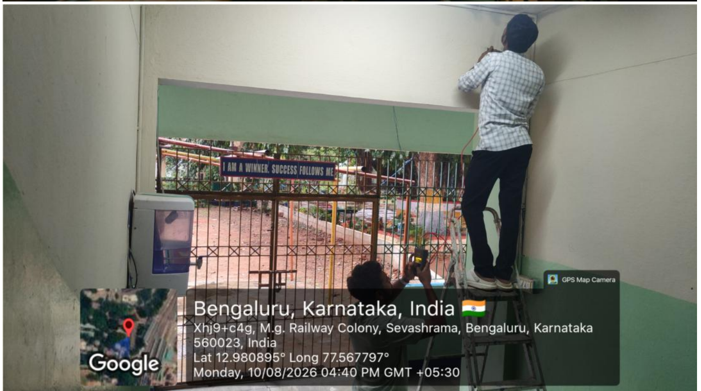
FIG. NO. 15& FIG.NO. 16: ULTRASONIC PULSE VELOCITY TEST AT SELECTED BEAM PM SHRI KENDRIYA VIDYALAYA, MG RAILWAY COLONY BENGALURU, 560023
