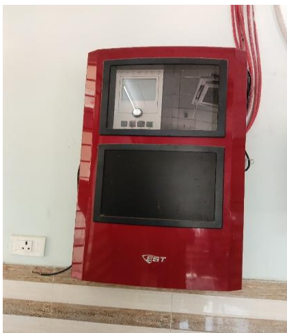
(FIRE ALARM CONTROL PANEL)
