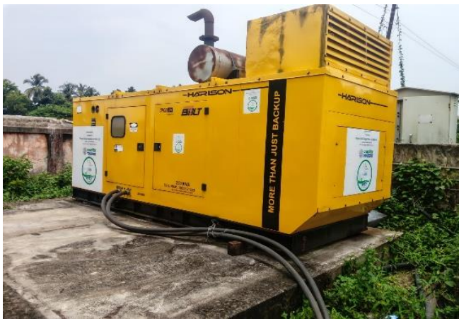
(BACK UP GENERATOR)
