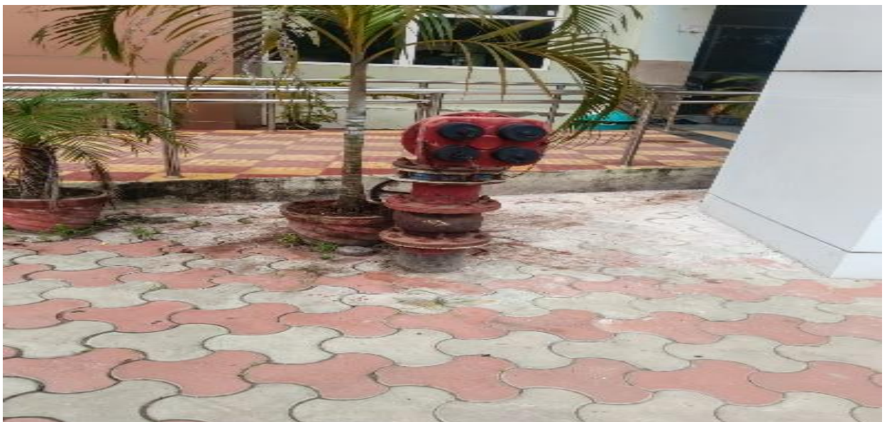
(4 WAY FIRE BRIGADE INLET WATER POINT)
