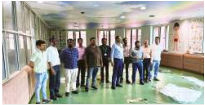
Executive Engineers (C), SCPMC CPWD, Mr Manohar Lal and Mr Mayank Saxena, inspecting the construction of the 'Creche' in room no 201 and 202, second floor, E block, Additional Building Complex
