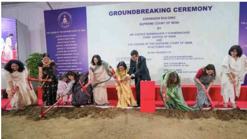
14 October 2024, Chief Justice of India, Dr D Y Chandrachud, along with Ms Kalpana Das and spouses of other sitting judges, at the “Groundbreaking Ceremony of Expansion Building”
