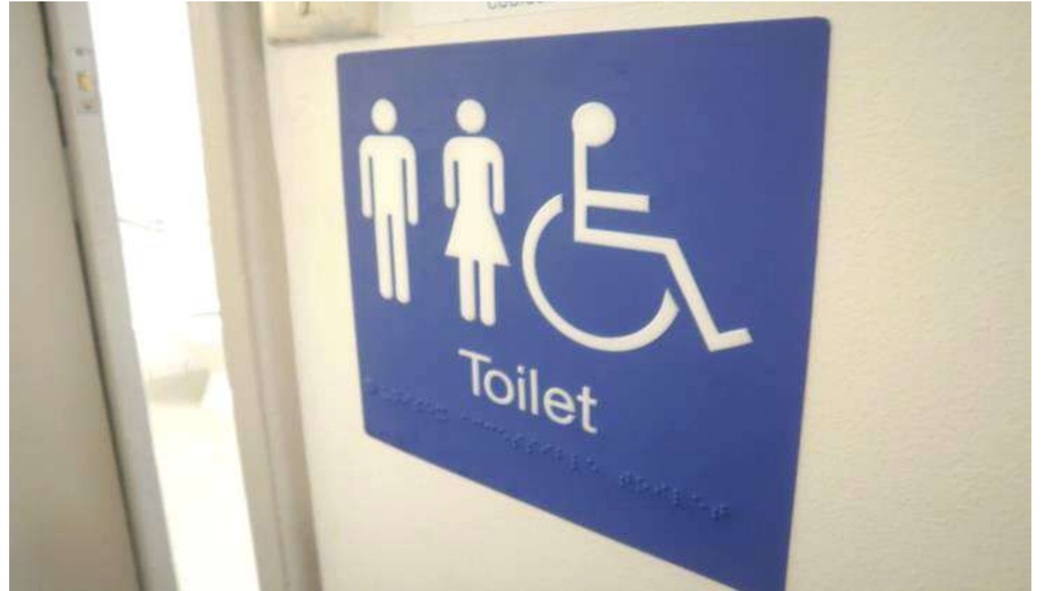
Good Practice - Signage Panels with textual, braille and pictographic information, high colour contrast
