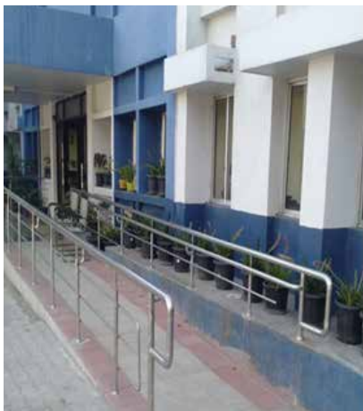
Ramp with double height handrails provided in Office of Accountant General, Kohima, Nagaland
