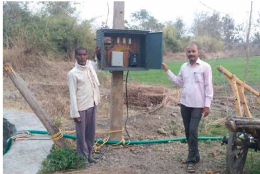
Electricity connection to agri-pumps.
