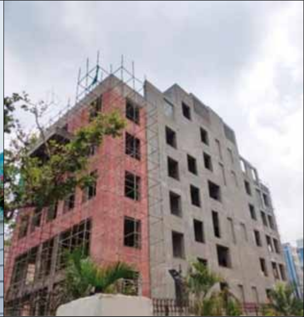
Construction of Office Building of Upper Yamuna River Board, Noida, Uttar Pradesh
