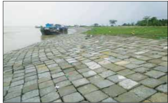
Protection of Majuli Island from flood and erosion of river Brahmaputra -Laying of Cement Concrete Block at Kamalabari Ghat, Majuli (Assam)
