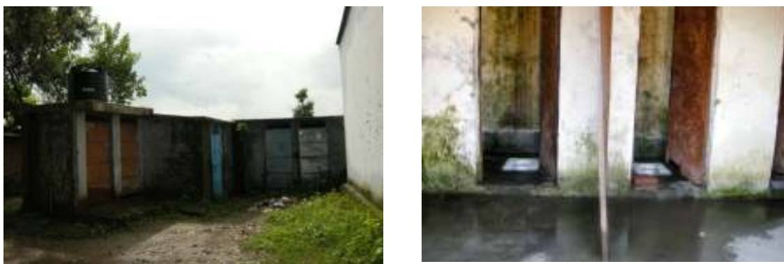
Picture 5.3-5.4 showing lack of O& M of School & public toilets
