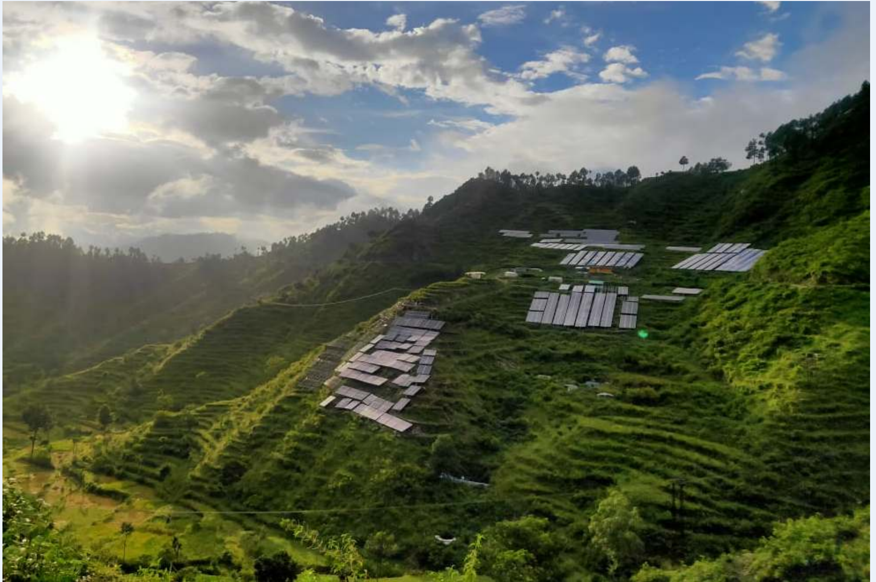
Solar Project of 900 KW installed at Village Odda, Block-Kot, Pauri
