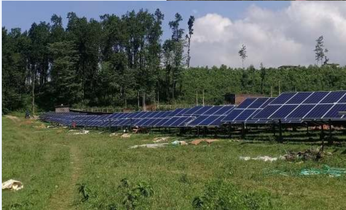
Solar Project of 400 KW installed at Dunga, Dehradun
