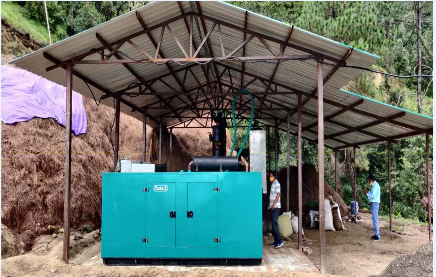
25 KW Plant installed in Didihat, Pithoragarh
