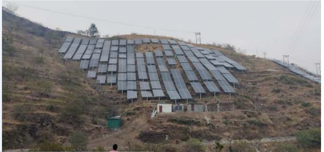
Solar Project of 1 MW installed at Landowne, Pauri Garhwal
