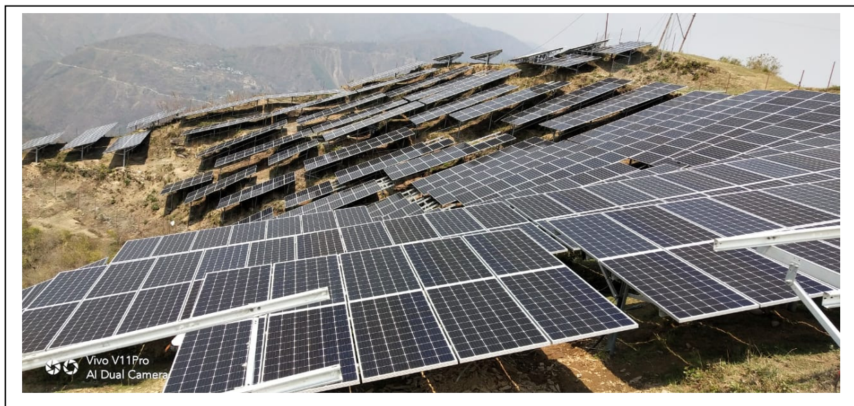
M/s ESCOBAR ENERGY PRIVATE LIMITED 1700 KW Solar Power Plant at Vill: Dhari, P.O. Satpuli, Distt. Pauri Garhwal, Uttarakhand Project Cost: 793.00 Lakh Employment: 6 persons
