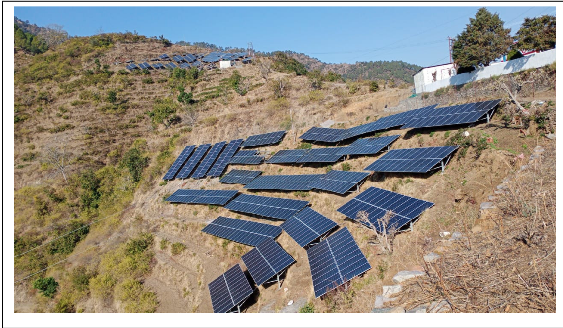
M/s Bisht & Company 200 KW Solar Power Plant at Village Goom, P.O. Amola, Pauri Garhwal Project Cost: 101.80 Lakh Employment: 2 persons
