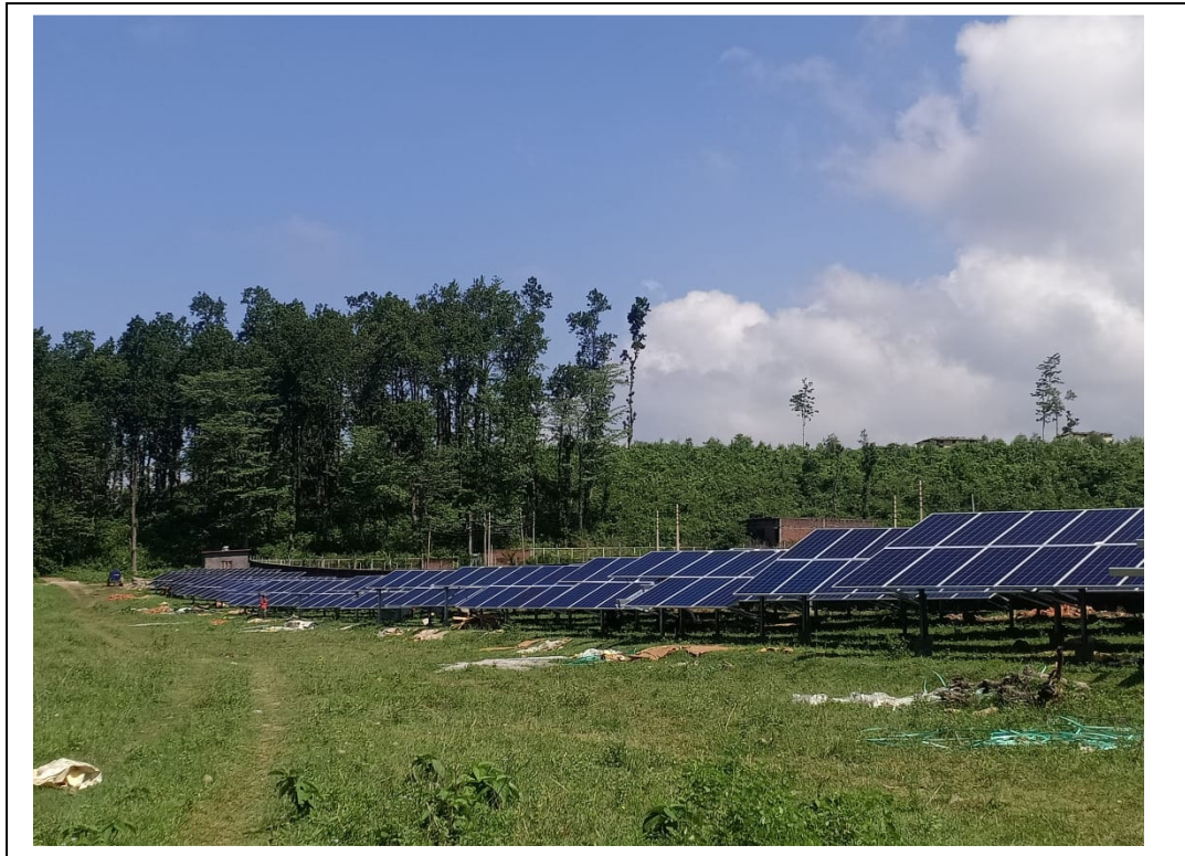
M/s Deepak Kumar 400 KW Solar Power Plant at Vill: Dunga, P.O. Bidholi, Dehradun Project Cost: 187.35 Lakh Employment: 2 persons
