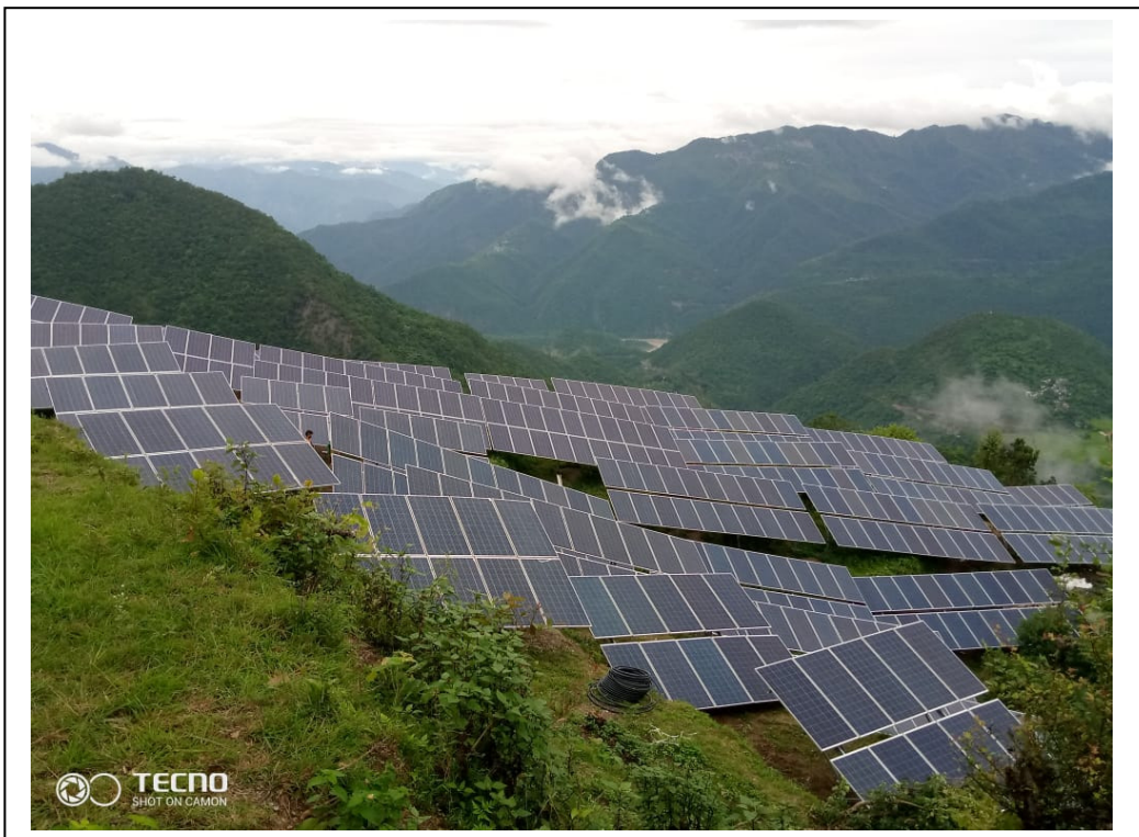
M/s Renu Bisht 200 KW Solar Power Plant at Village Goom, P.O. Amola, Pauri Garhwal Project Cost: 101.80 Lakh Employment: 2 persons
