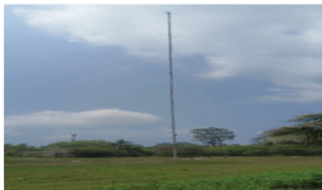
Fig. 9.13: 100m WMS installed at Bharatpur
