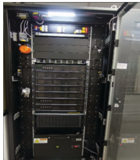
Figure 7.6 HPC Server for CFD at IIT Roorkee
