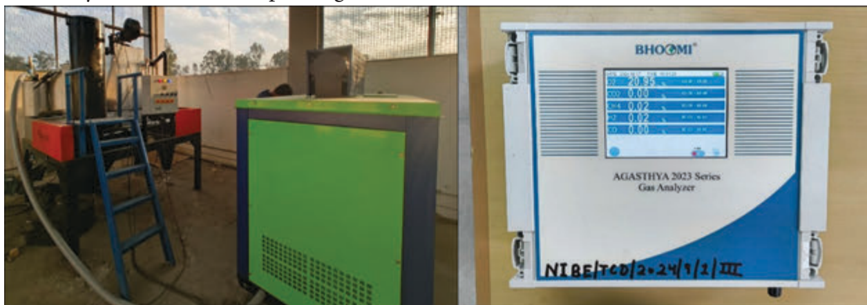
Figure 7.9 (Left) Biomass Downdraft gasifier with Gen set (10KVA); Producer gas analyser (Right)
