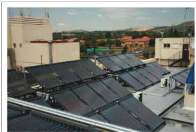
Figure 15 SWHS installed in Union Hospital in Gauteng, South Africa
