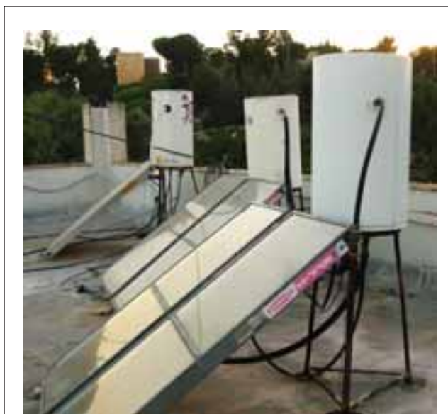
Figure 2 Flat plate solar water heaters on residential rooftops 3
