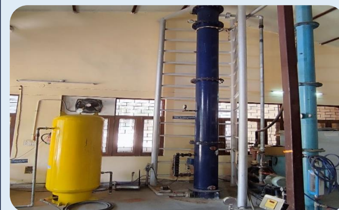
Biogas upgradation system at BDTC IIT Delhi
