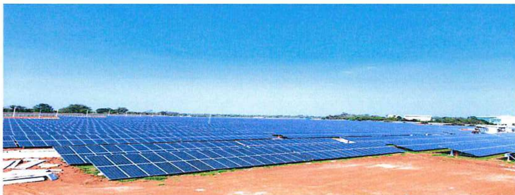
Fig. 10.20: 10 MW solar project in DRDO Karnataka
