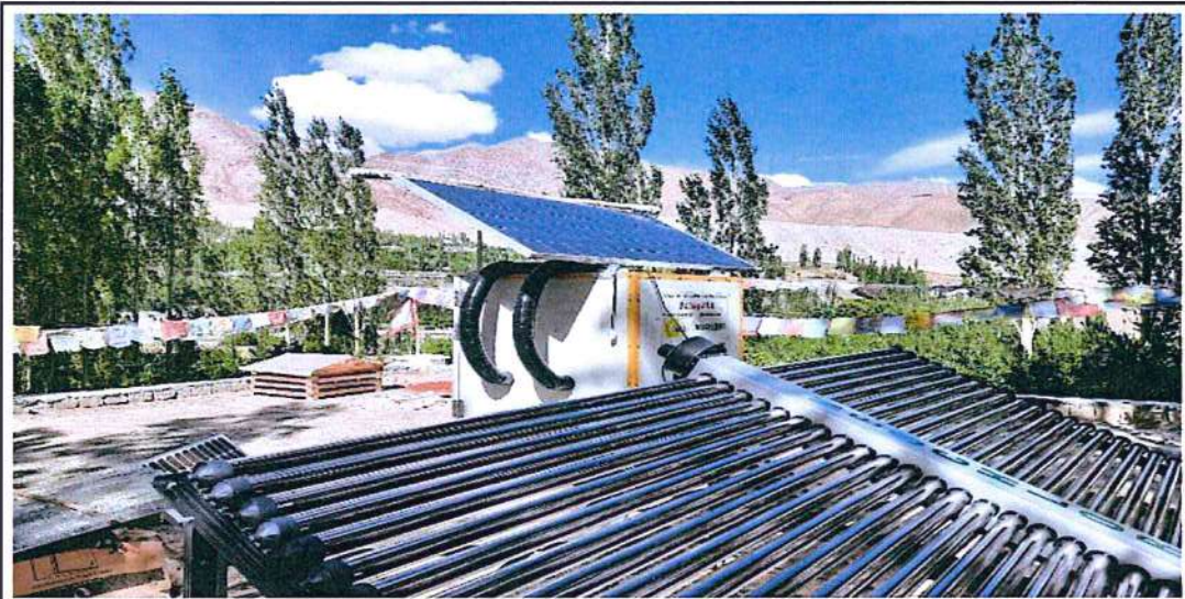
Fig. 10.9 Solar Dryer cum Space Heating unit in Ladakh
