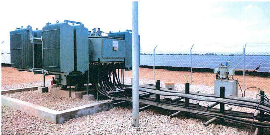
Fig. 10.19: 50 MW solar project in Rajasthan under ISTS I
