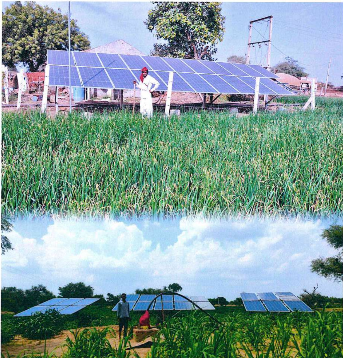
Solar Pump installed in Rajasthan
