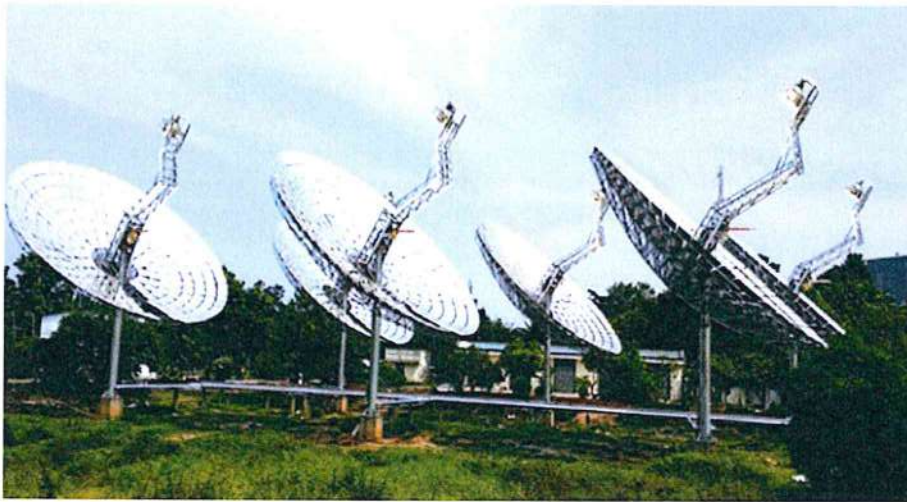
Fig. 3.4: CST-based Solar Project at M/s. Kasturi Estates Pvt. Ltd., Chennai, Tamil Nadu
