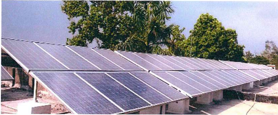
Fig. 1.1: Roof Top Solar Power Plants increase the efficient utilisation of Power
