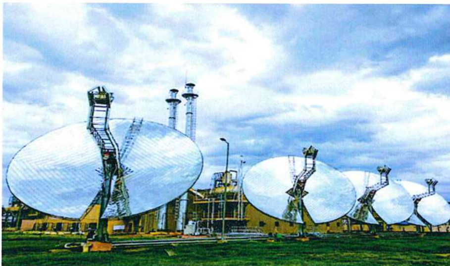
Fig. 3.5: CST based solar project at M/s. Mondelez India Foods Pvt. Ltd., A.P.
