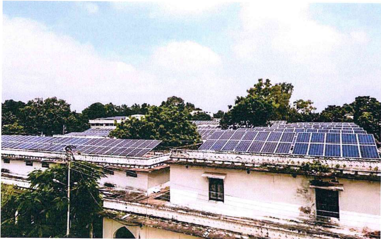
494 kWp Rooftop Solar PV Power Plant at University of Lucknow, Uttar Pradesh
