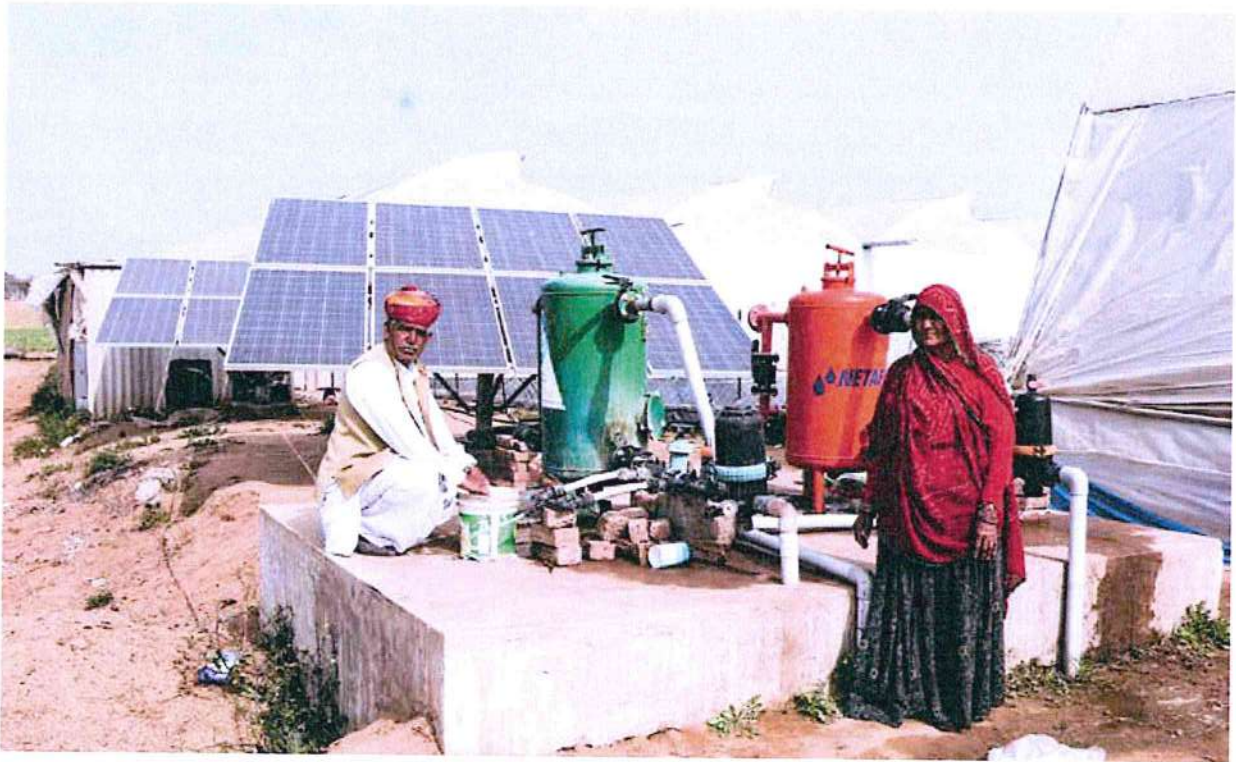
5 HP solar pump installed in Sambhar, Jaipur District, Rajasthan
