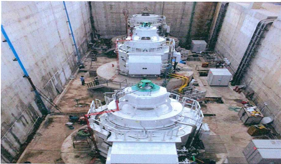
Fig.4.6: TG sets of Baitarani SHP (24 MW) commissioned in August 2020 in Keonjhar District of Odisha
