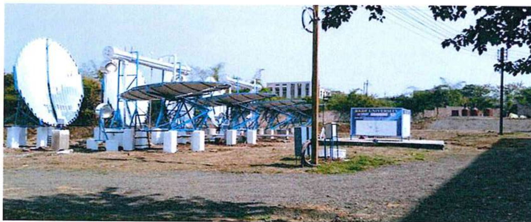
Fig. 7.10 : Solar Thermal Power Plant at RKD Foundation University
