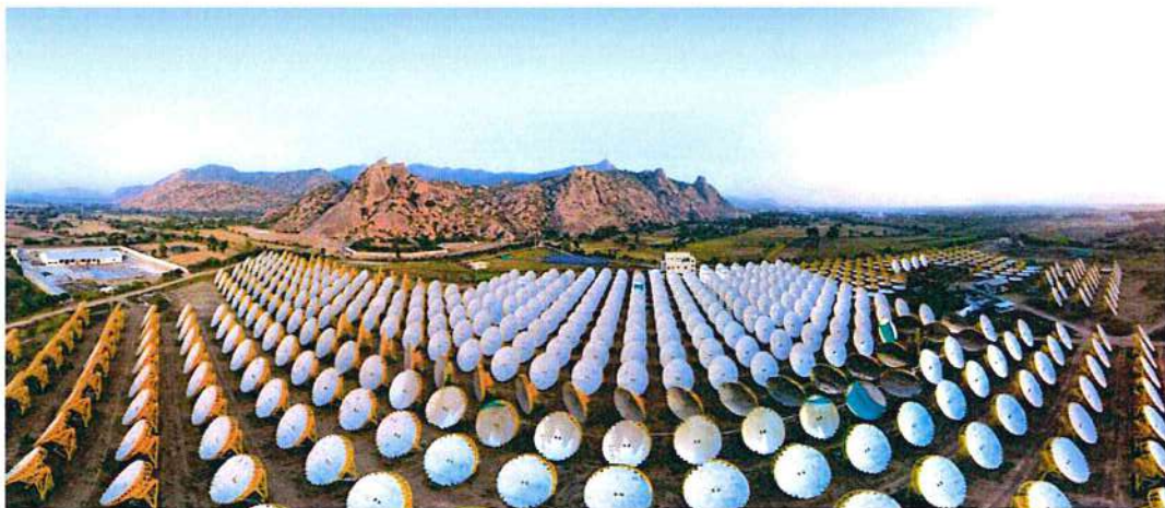
Fig. 7.7: One MWe (3.5 MWth) Solar Thermal Power plant based on Parabolic Dish Solar concentrators
