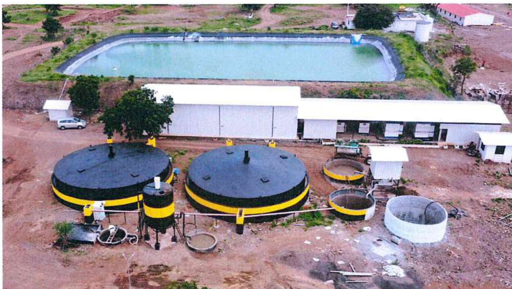
Fig. 5.1 : Biogas Power-Off-grid Project (S&P Feeds Pvt. Ltd., Vill Post- Thengoda, Block Taluka-Baglan, District-Nashik-423301 (Maharashtra)
