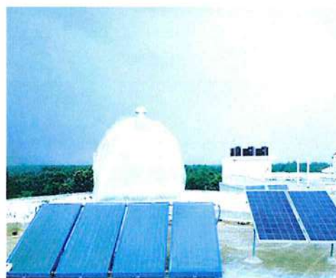
Fig. 7.14: Mixed-mode Solar Dryer installed for rubber sheet drying
