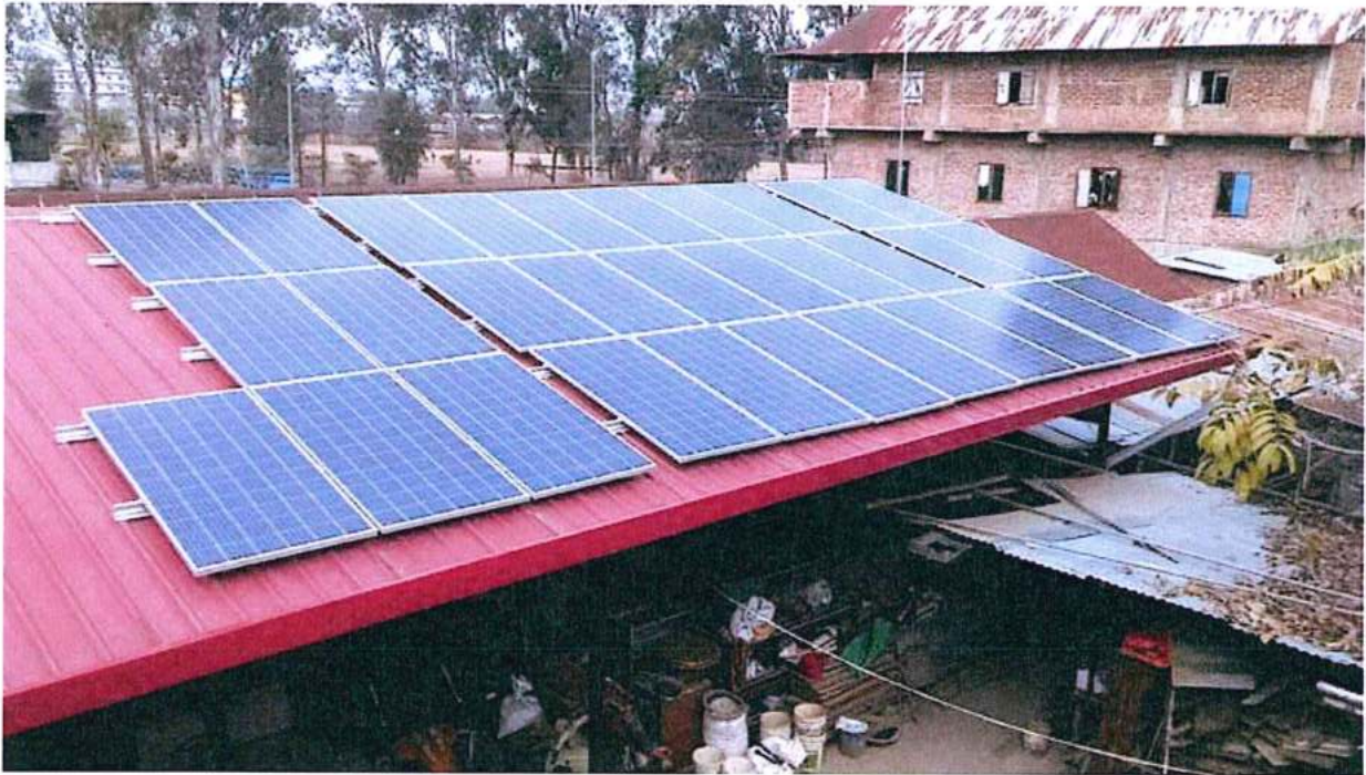
10 kW Residential Grid Connected Solar Rooftop Plant at Koirengai, Imphal, Manipur
