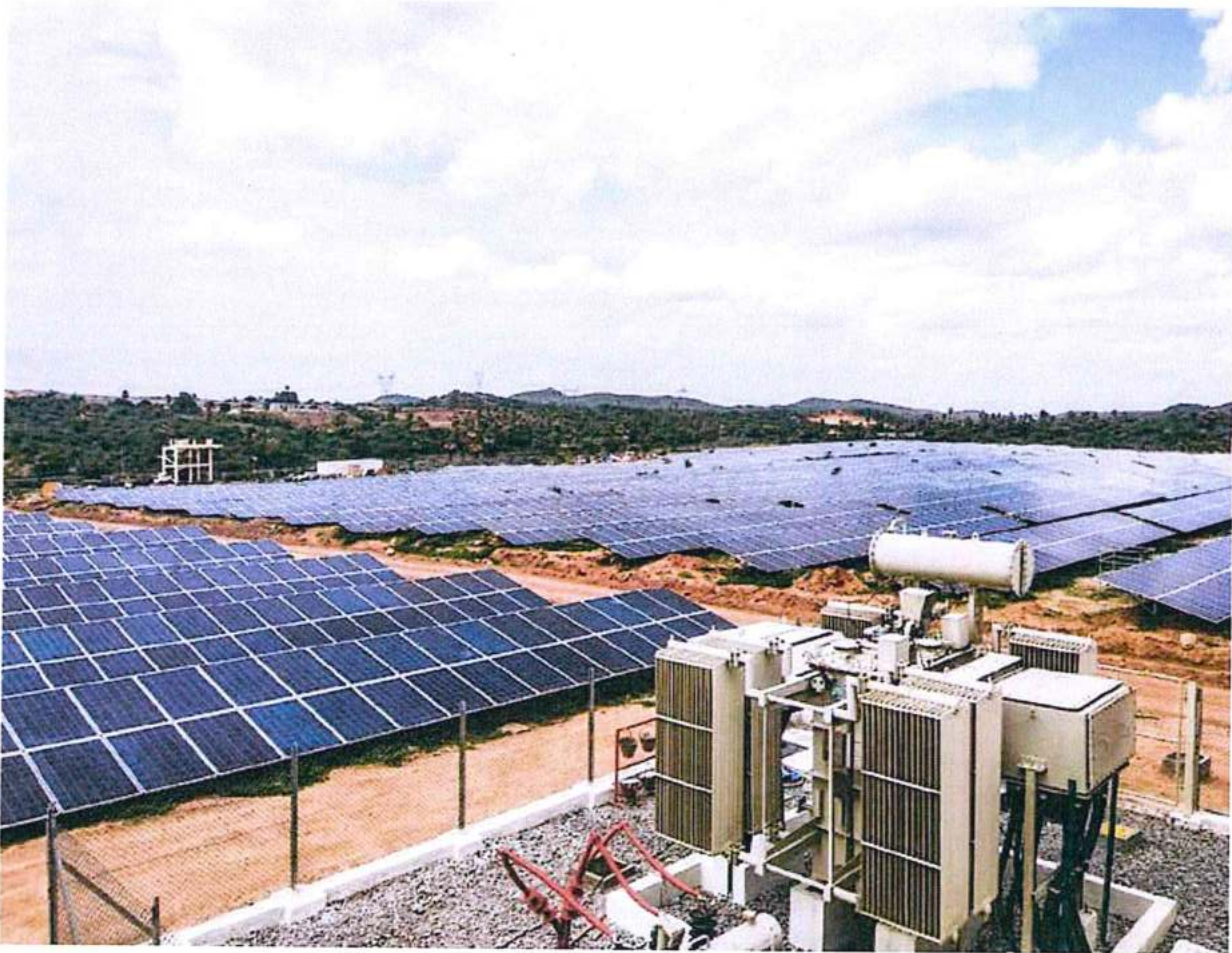
5 MW Solar PV Project in Ibrahimpatnam
