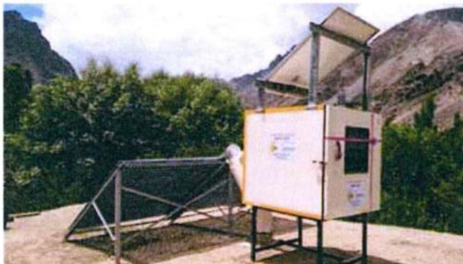
Installation of Solar Apricot Dryer cum Space Heating System at Minjee Village, Kargil District
