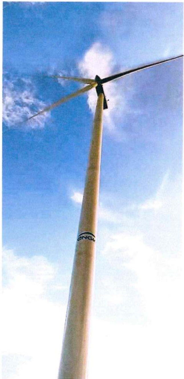
Wind Turbine in SECI tendered project in Tamil Nadu
