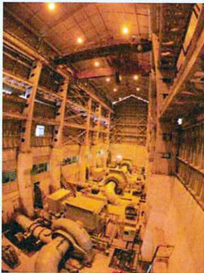
DIKSHI 24 MW SHP-Power House
