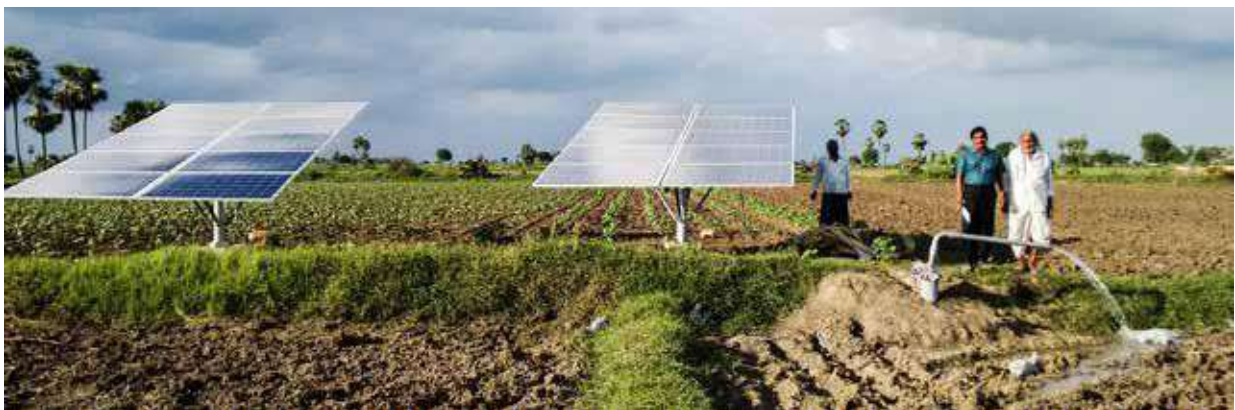
5 HP Solar Pump installed in the State of Andhra Pradesh
