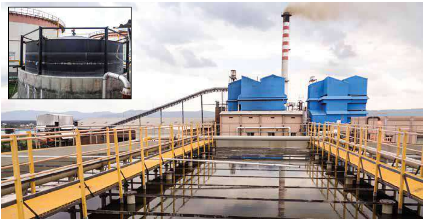
24000 m 3 /day Biogas generation plant from Starch and allied Manufacturing Unit of Ms Gujarat Ambuja Exports Ltd. at Jalgoan, Maharashtra. Inset shows Digester Overview
