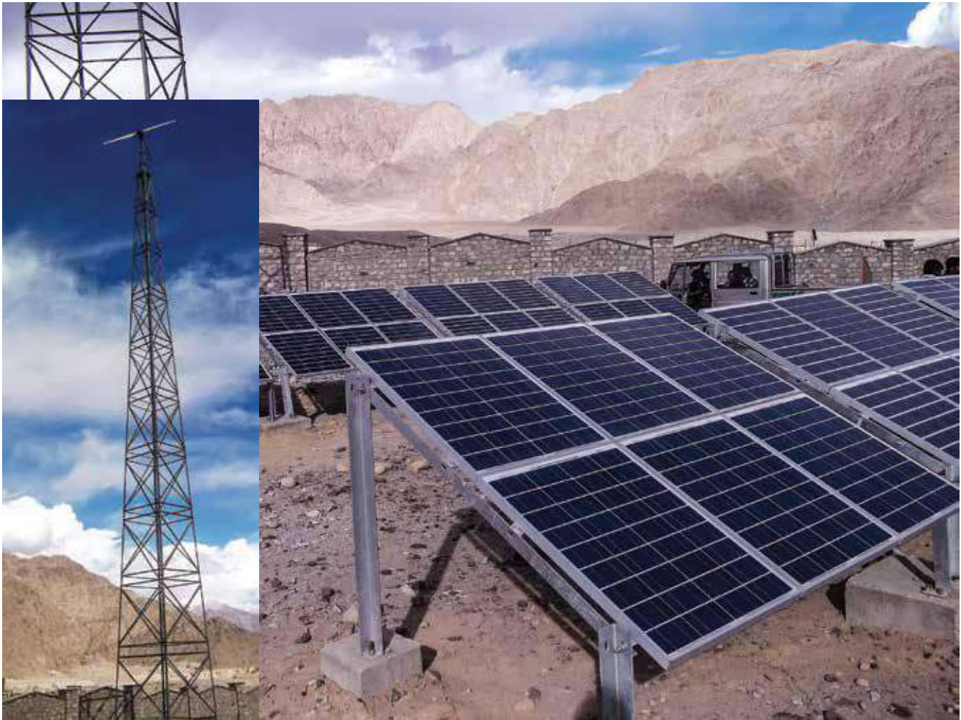
Small Wind and Solar PV Hybrid System at Puga, Ladakh, J&K
