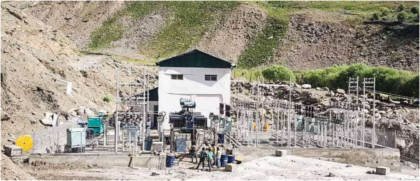
1.5 MW Sangrah SHP in Kargil district of Jammu & Kashmir under 'Ladakh Renewable Energy Initiative'
