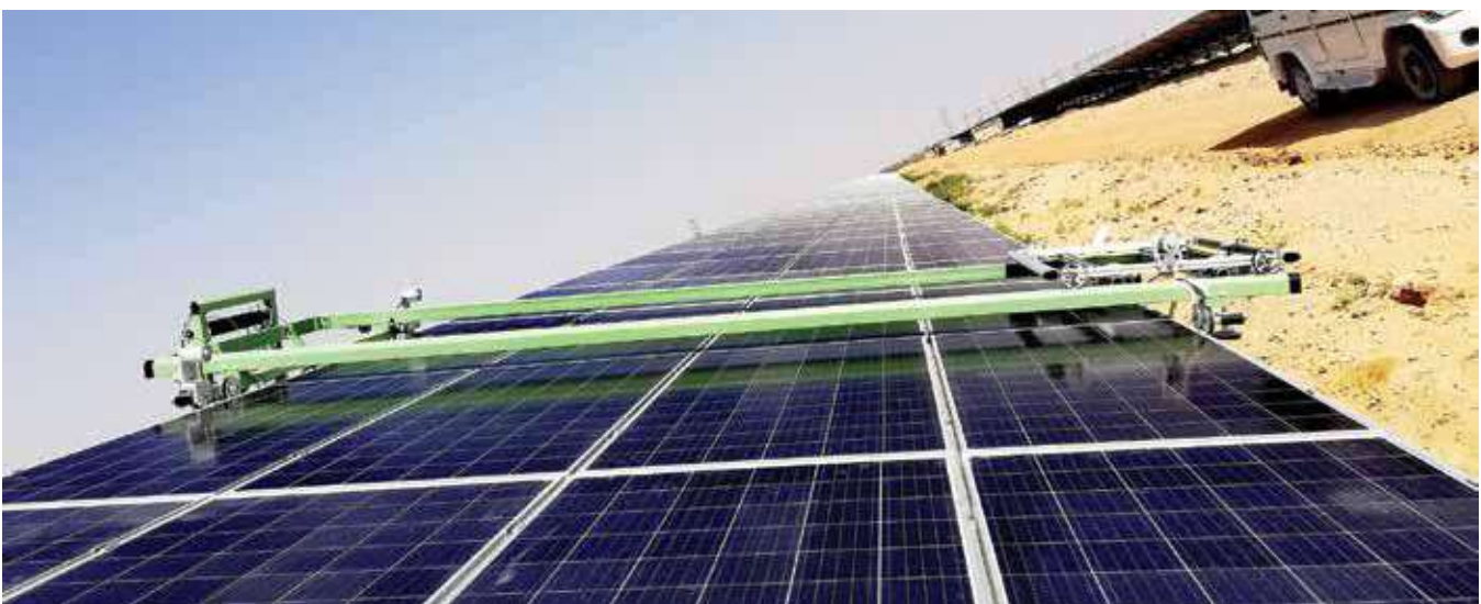
50 MW SB Energy Two Pot Ltd, Bhadla Ph-IV Solar Park, Jodhpur
