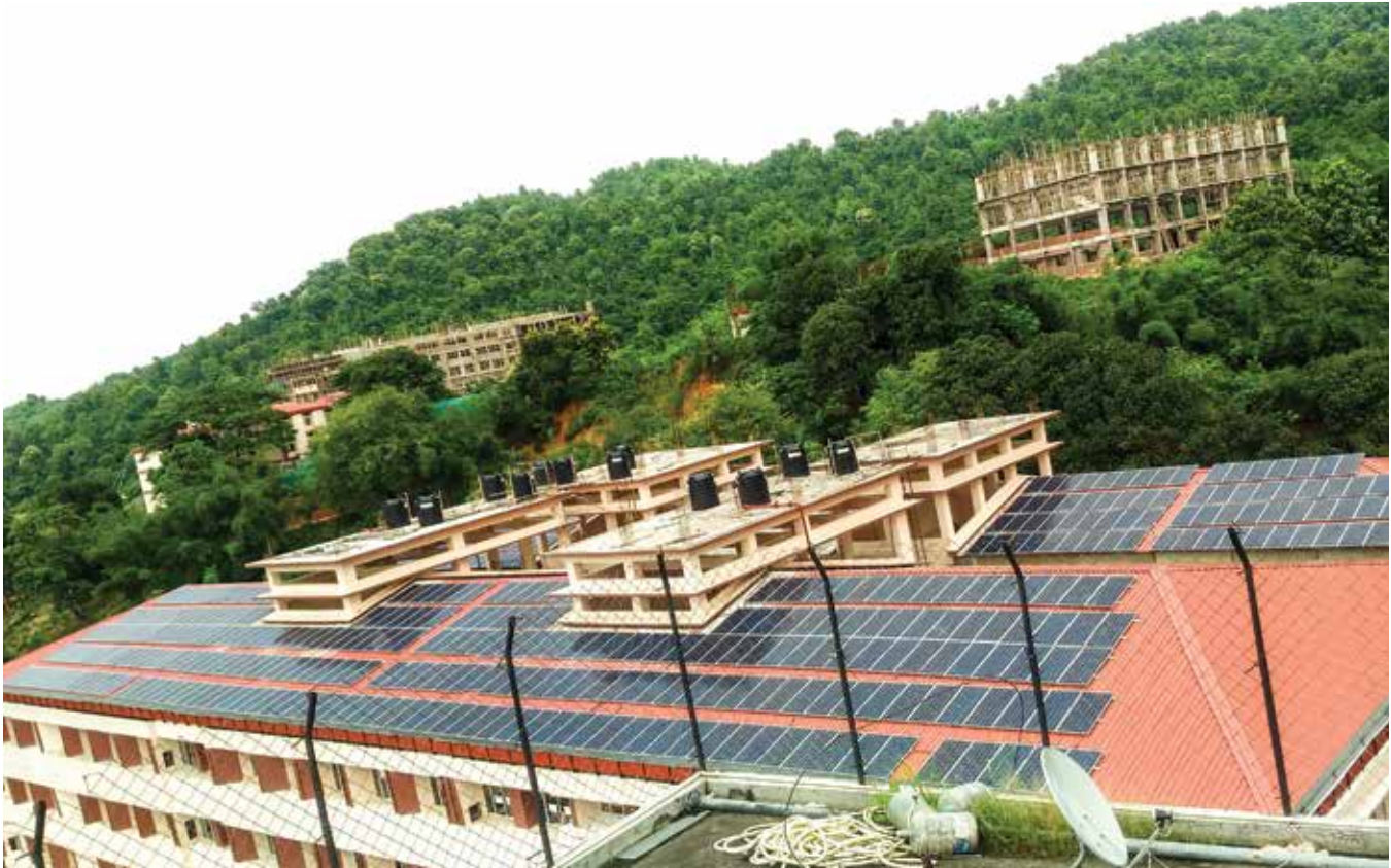
200 kWp Rooftop Solar Plant installed in Down Town University, Guwahati, Assam
