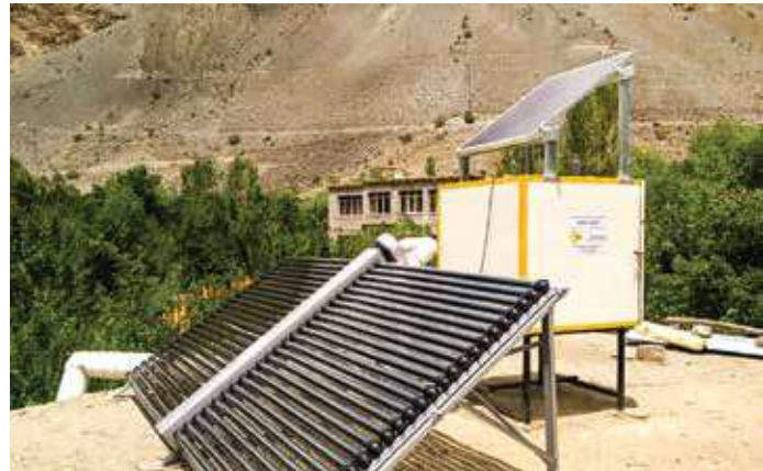
Installation of Solar Apricot Dryer cum Space Heating System at Minjee Village, Kargil District
