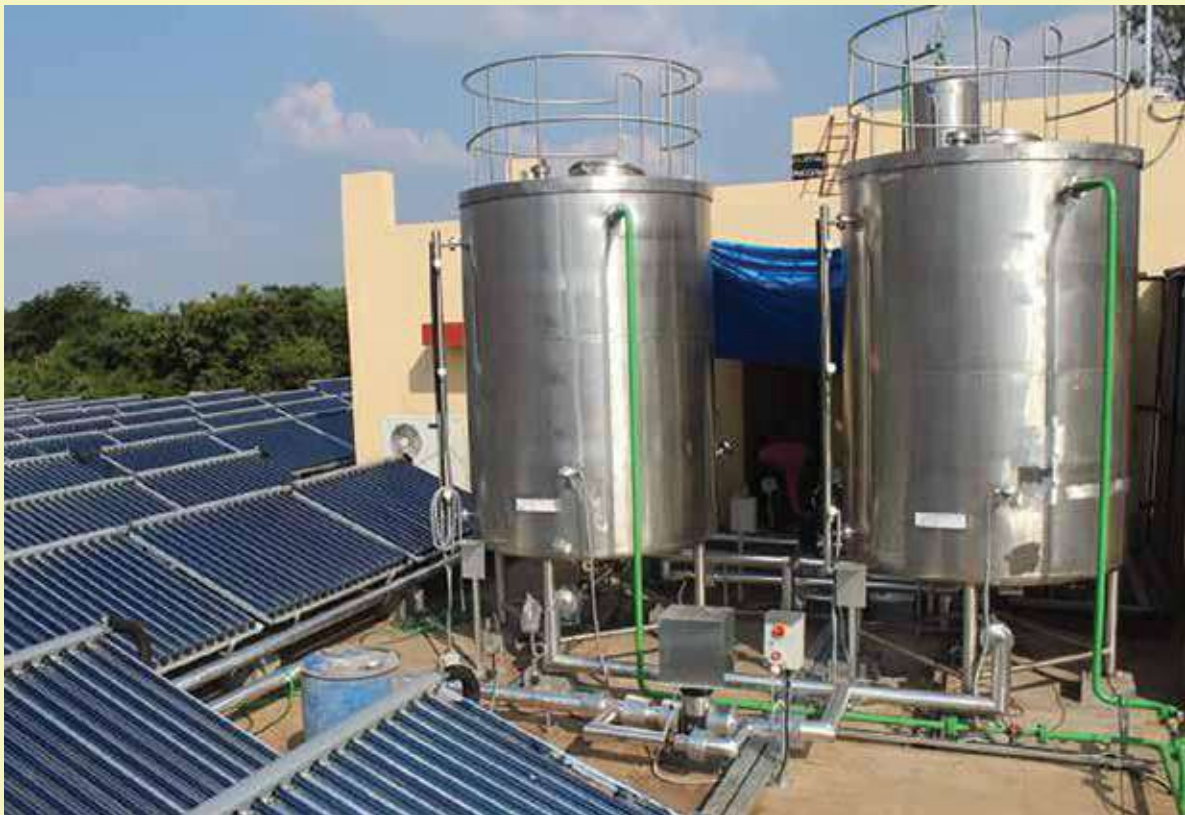
Solar Field and storage tanks at M/s. Raichur, Bellary & Koppal Districts Co-operative Milk Union Ltd.
