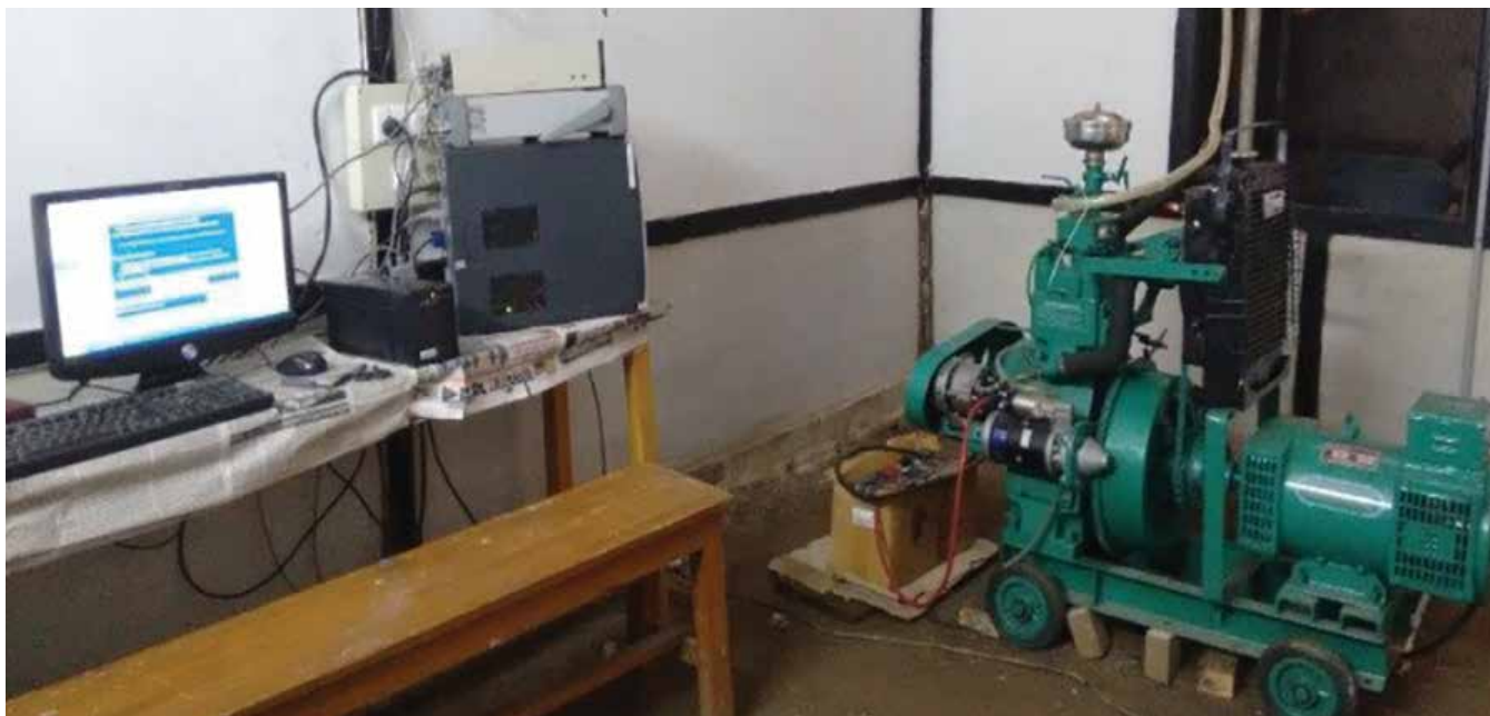
Biogas generator and data monitoring system at IIT Guwahati
