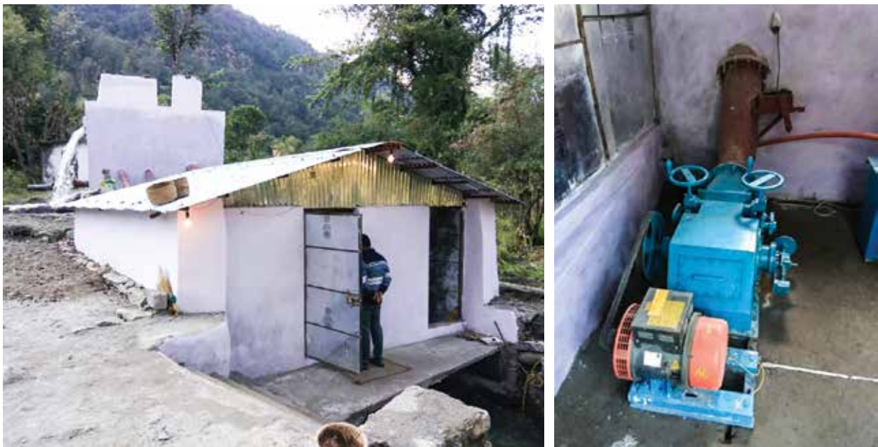
5.0 kW Modified Cross flow Turbine installed at Mandal village, Chamoli district, Uttarakhand
