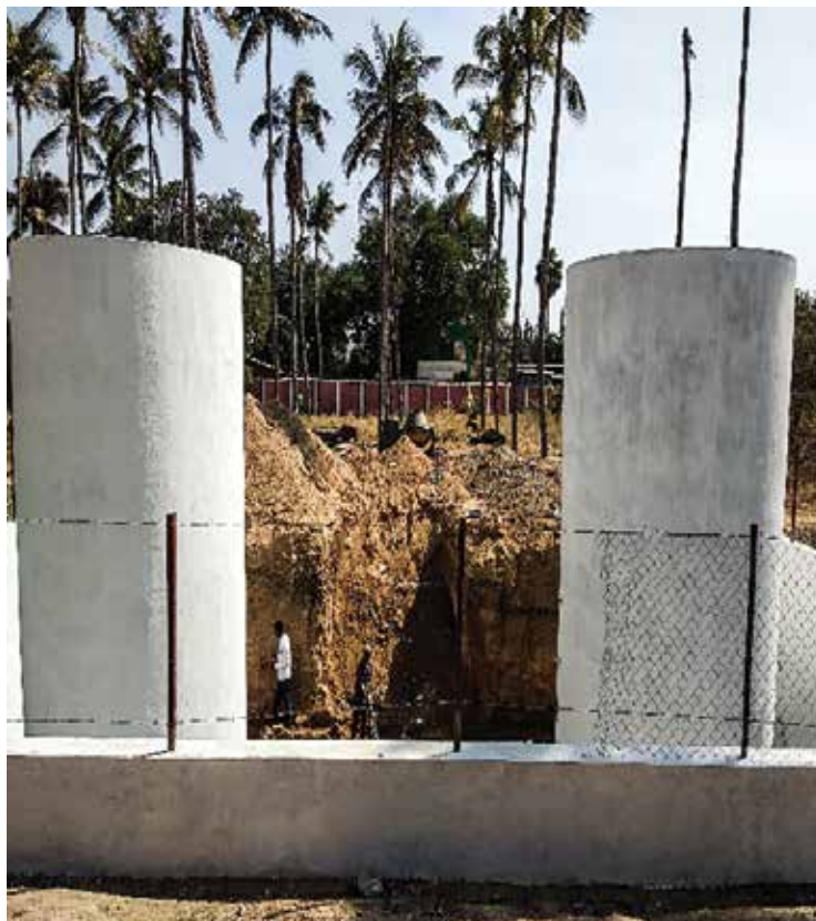
High rate reactors and Hybrid high rate reactors with masonry structure installed at TNAU boys hostel
