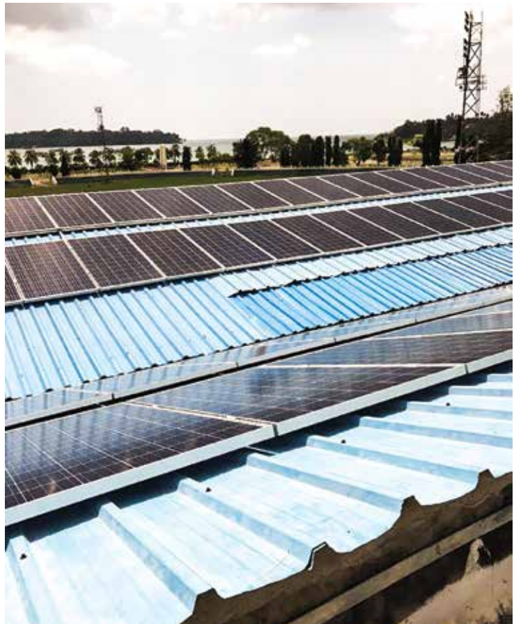
1 MW Solar PV Power Plant established at Port Blair, Andaman & Nicobar Islands
