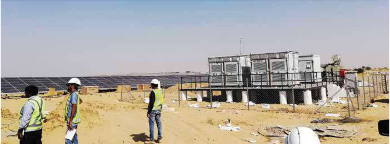
50 MW Phelan Energy Pot Ltd, Bhadla Ph-IV, Jodhpur
