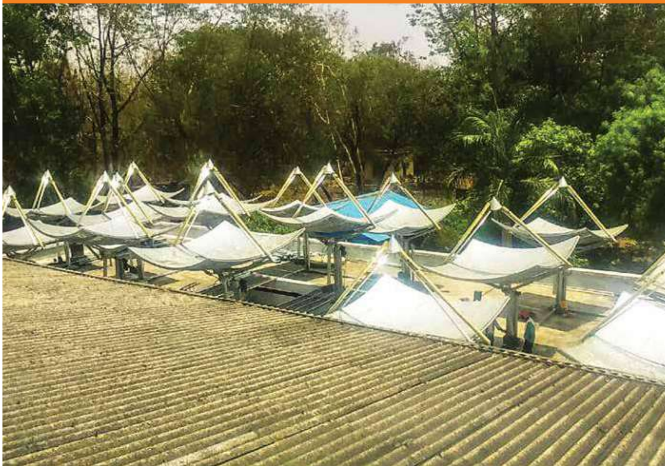
Parabolic dish based CST system installed at Indian Ordnance Factory, Nagpur.
