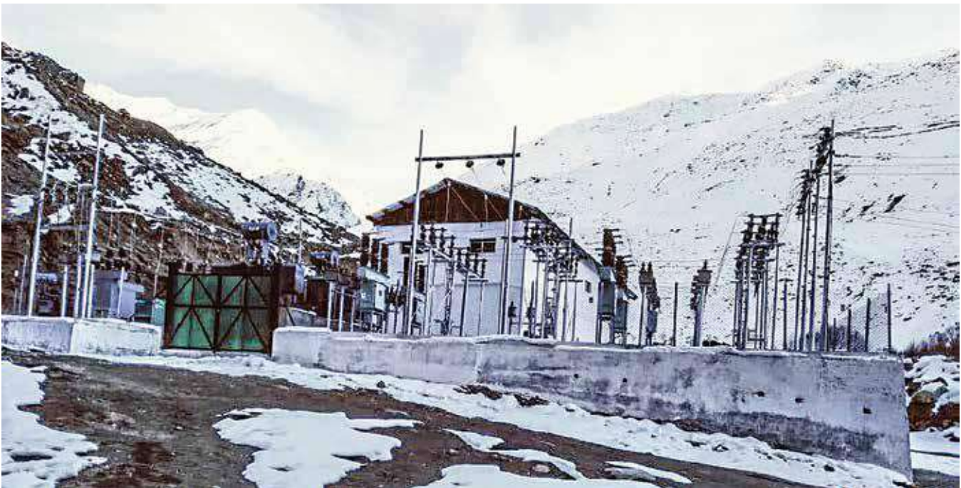
1.0 MW Chilong SHP in Kargil district of Jammu & Kashmir under 'Ladakh Renewable Energy Initiative'
