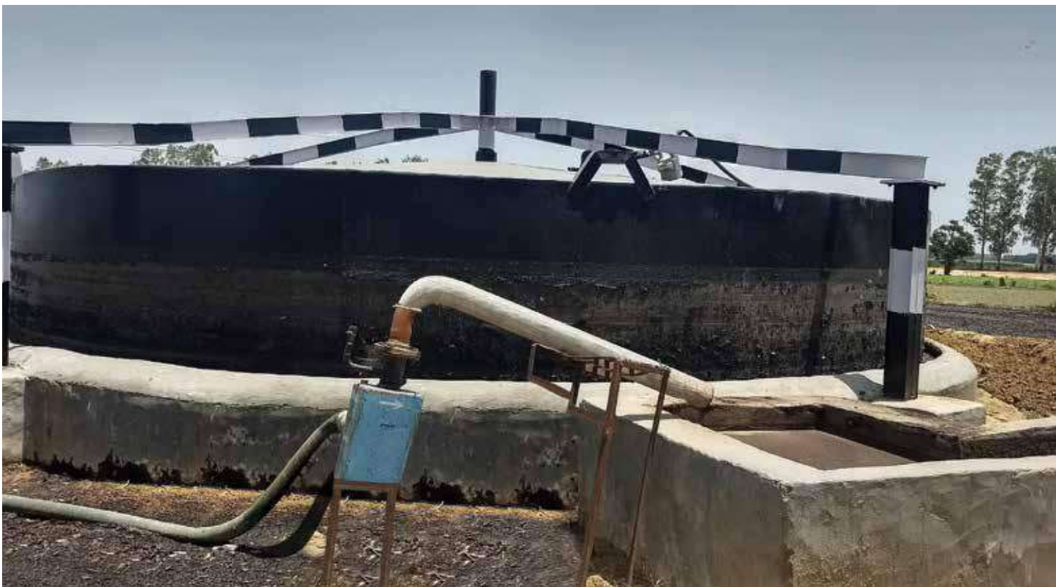
Biogas Power Project of 40 kW (350 m 3 ) installed at VPO-Gehlewal, Samrala, Ludhiana, Punjab
