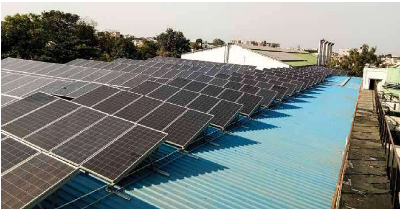
700 kWp Grid Connected Rooftop power plant project at Ahmedabad Airport, Gujarat
