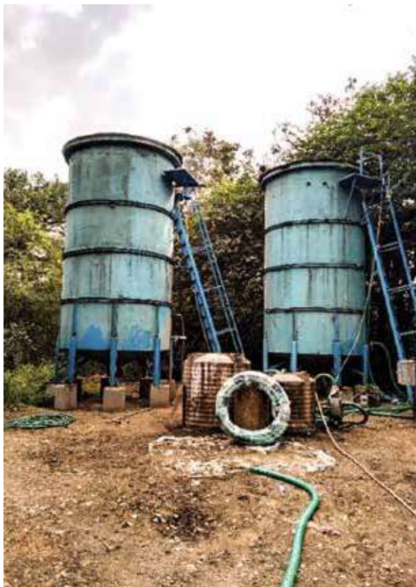
High rate reactors and Hybrid high rate reactors with steel GLS installed at TNAU ladies hostel
