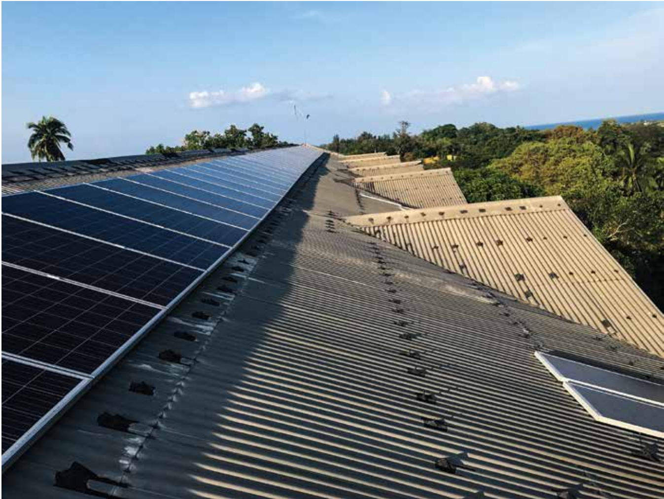
1 MW Solar PV Power Plant established at Port Blair, Andaman & Nicobar Islands
