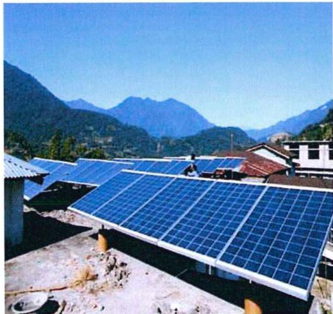
Solar Photovoltaic Power plant and Solar Water Heating Systems at District hospital in Arunachal Pradesh
