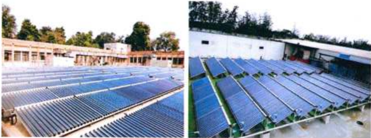
Fig. 3.CPC Collectors at GTPS, Gujarat and HUL, Amlī
