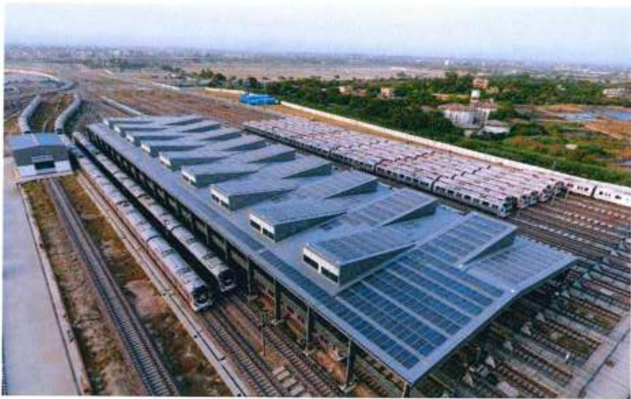
Grid connected solar rooftop plants of 387 kWp installed at Mukundpur Metro Station of Delhi Metro Rail Corporation Ltd.
