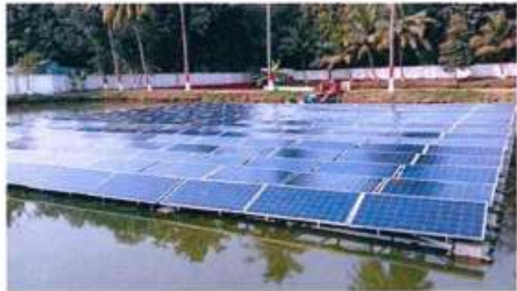
Installation of 60kWp Floating Pond Top Solar Power Plant at Hon'ble Governor House in Bihar
