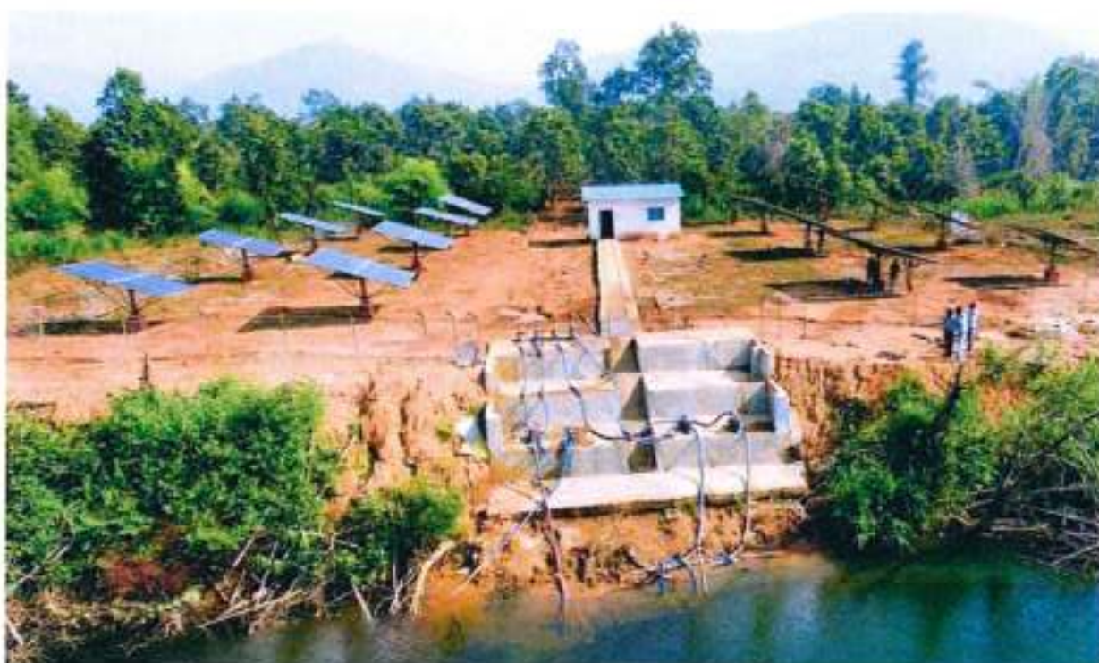
Community Solar Pump Systems installed at Kulhadighat Distt. Gariyahandh, Chhattisgarh
