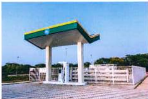
Hydrogen facility at NISE
