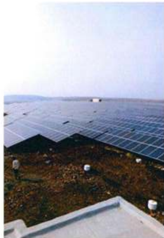
10 MW Solar Power Project in Maharashtra
