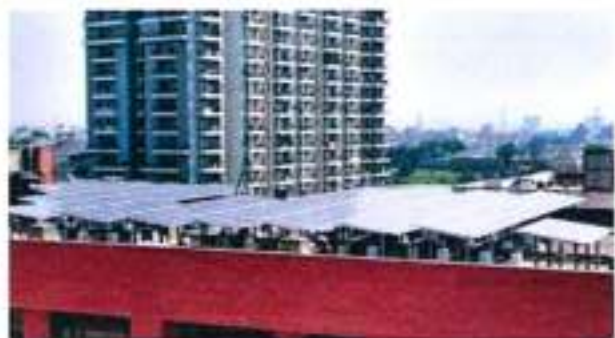
Grid connected solar rooftop plant of 170 kWp installed by SECI at Seth Anandram Jaipuria Education Society, Jaipuria Institute of Management, Indrapuram, Ghaziabad, Uttar Pradesh
