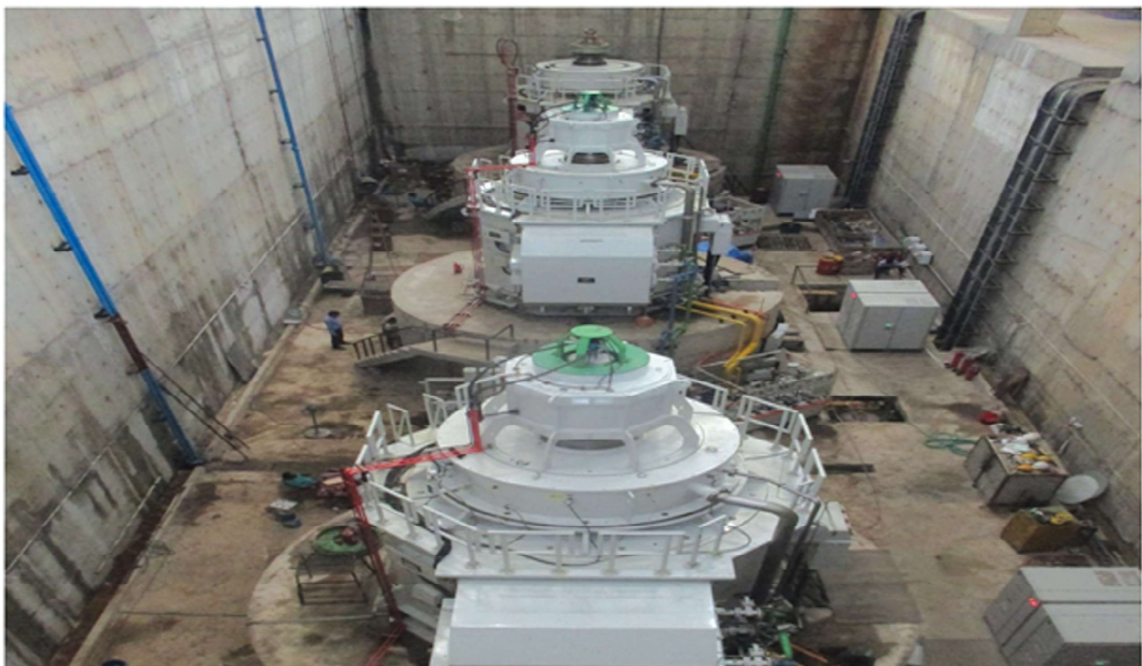
Fig.4.6: TG sets of Baitarani SHP (24 MW) commissioned in August 2020 in Keonjhar District of Odisha
