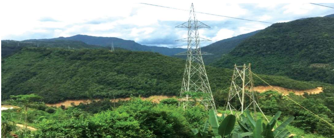
Fig. 8.1: Transmission System in 20 MW Vankal Solar Park in Mizoram
