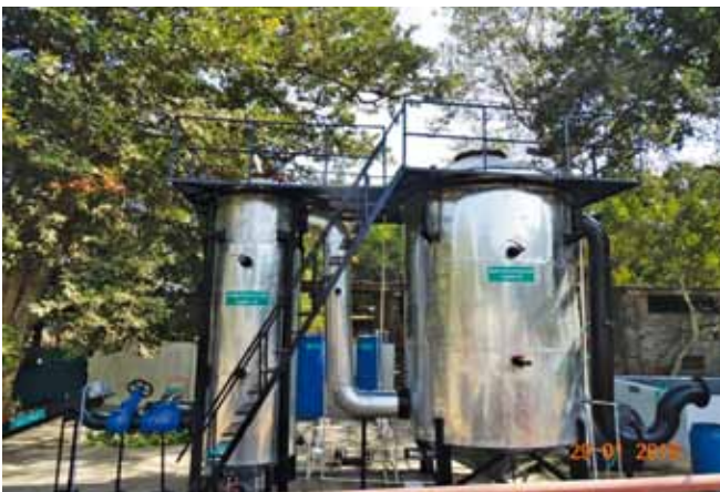
Biomethanation plant at SPRERI, Gujarat
