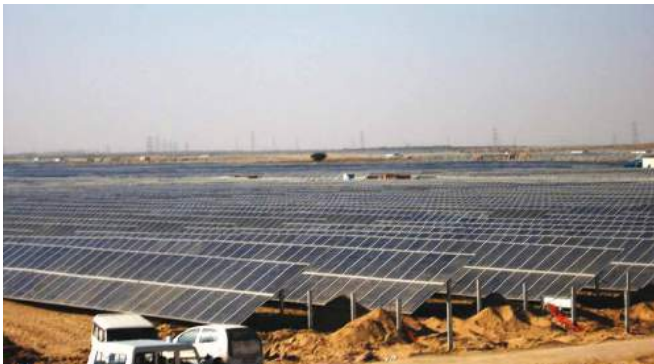
Solar plant being Developed by NTPC in Bhadla Solar Park Phase-II
