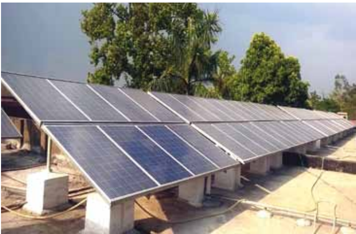
50 KW Rooftop SPVPP Installed at Collectorate Building, Korba, Chhattisgarh
