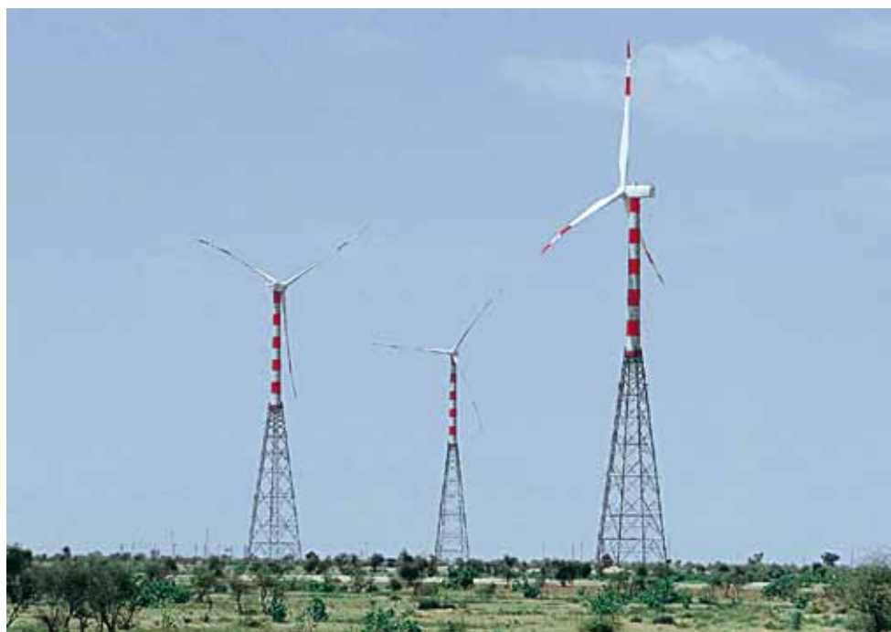
50.4 MW hybrid tower wind farm in Rajasthan
