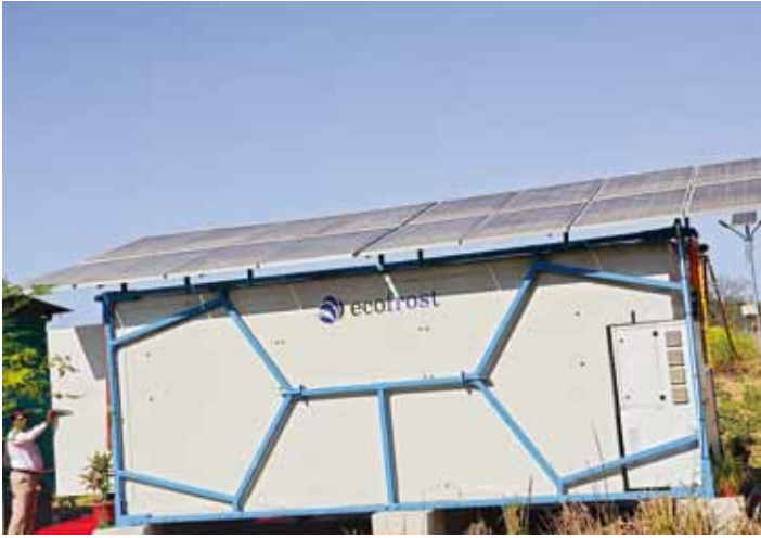
Solar Cold Storage system installed at Jagdalpur, Chhattisgarh
