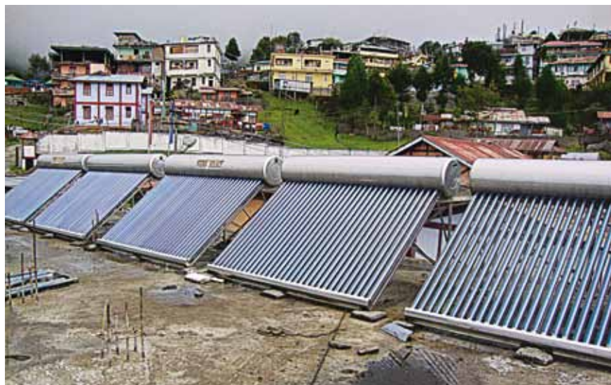
1000 LPD Water Heating System in Tawang, Arunachal Pradesh
