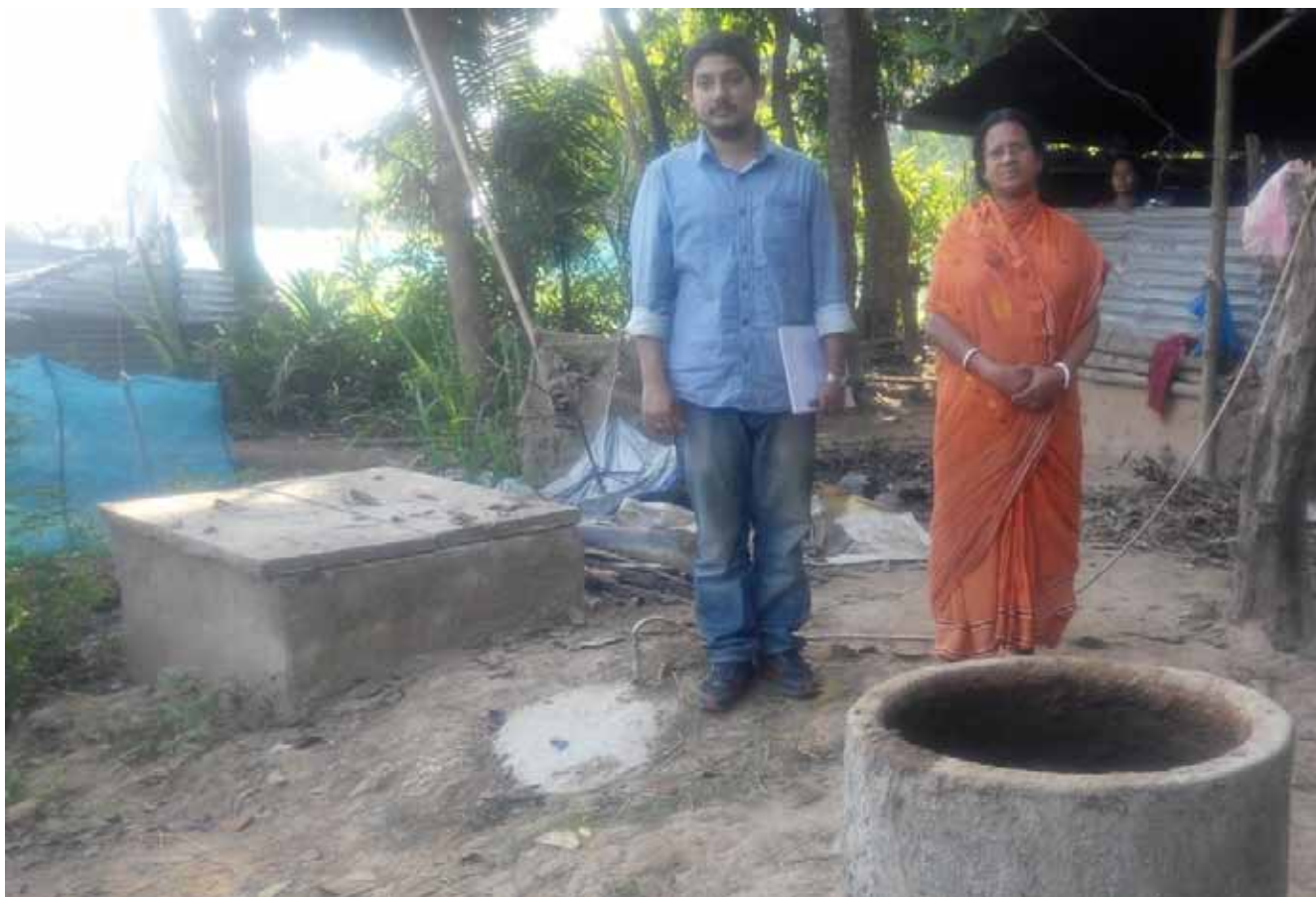
Deenabandhu Biogas Plant installed for beneficiary - Shri. Sudhir Das at village-Baidyamura, Nalchar RD Block, Tripura
