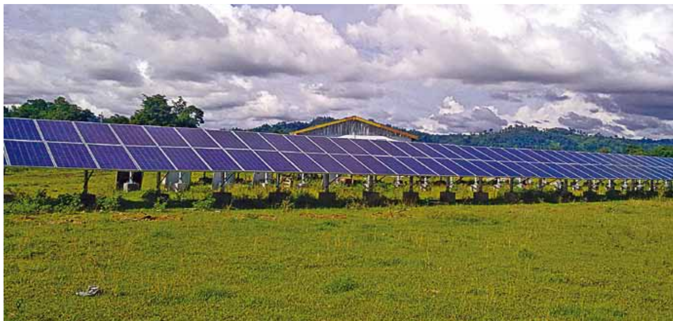
100 kW Solar Power Plant at Diyun
