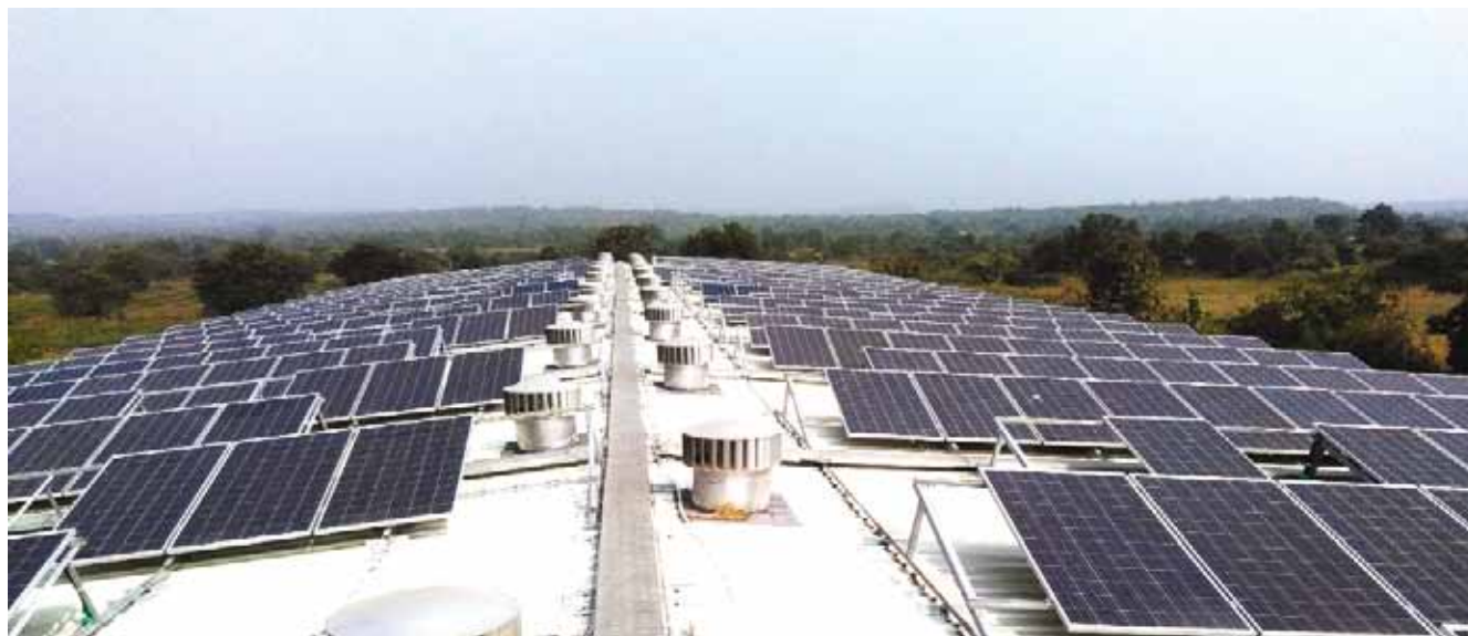
198 kWp grid connected solar rooftop plant at Pitambera Polymers Industries Pvt Ltd, Maharashtra
