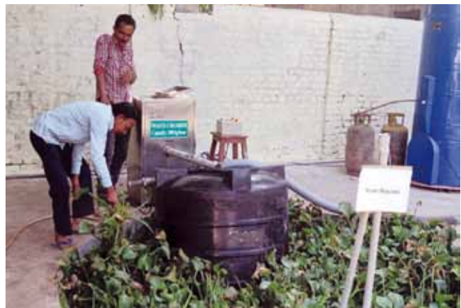
Crusher and feed preparation tank with submersible pump at SPRERI, Gujarat
