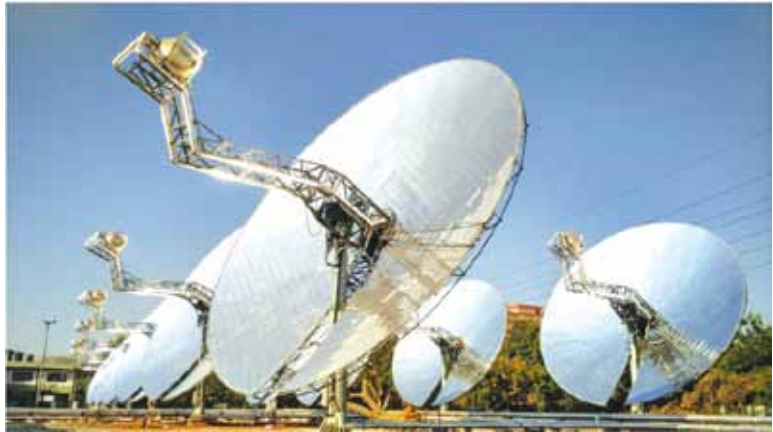
Installation of 1520 sq. m of Paraboloid Dish at Mother Dairy, New Delhi
