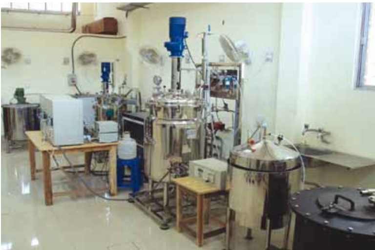
BIOMETHANE PILOT PLANT installed at IIT Kharagpur under lab and library upgradation component of HRD programme
