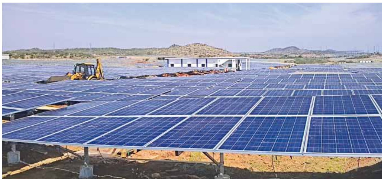
Solar Modules at the 250 MW Solar Park at Ananthapuramu, Andhra Pradesh
