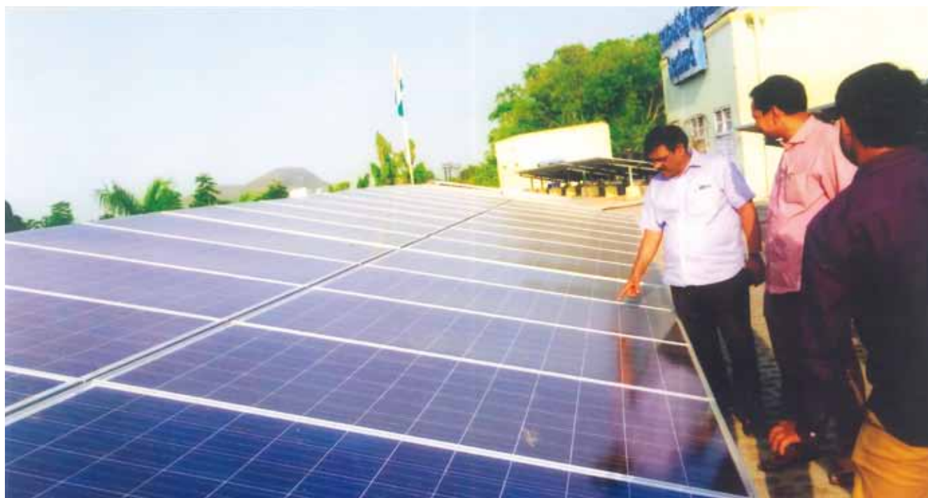
100 kWp Grid Connected Solar rooftop Power Plant at Municipal Office & Council Hall Building, Vijayawada, Andhra Pradesh
