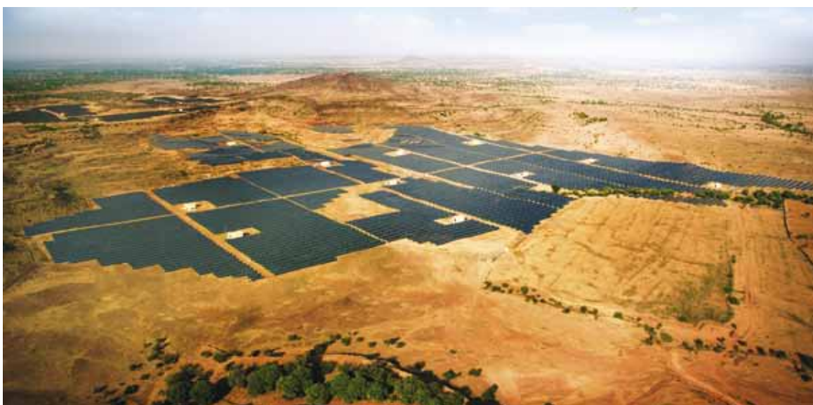
40 MW Project in Rajasthan commissioned under 750 MW VGF Scheme
