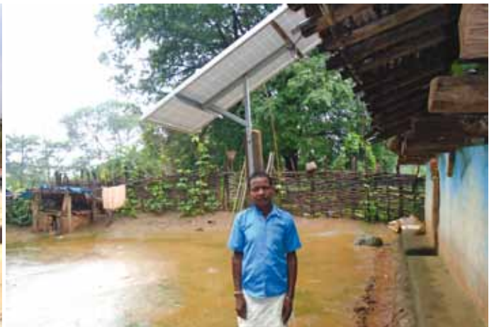
Solar Home Lighting system installed at Distt. Sukma, Jagdalpur, Chhattisgarh
