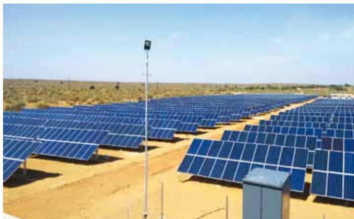
5 MW Project at Rajasthan
