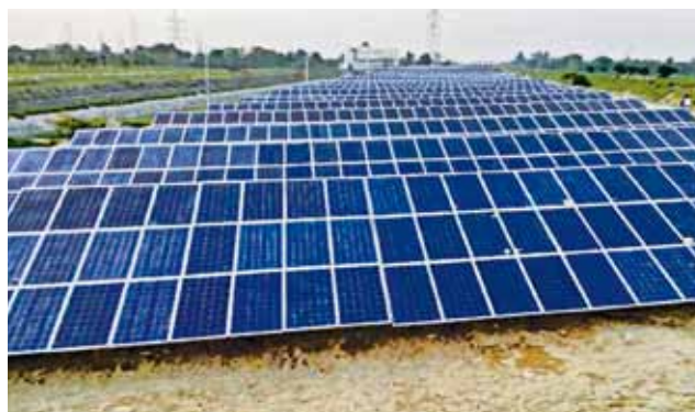
Canal Bank Solar Power project at Teesta Canal Full Stage -II Hydro Electric Power Station of WBSEDCL, Haptiagach, Block - Chopra, Dist. - Uttar Dinajpur, West Bengal.
