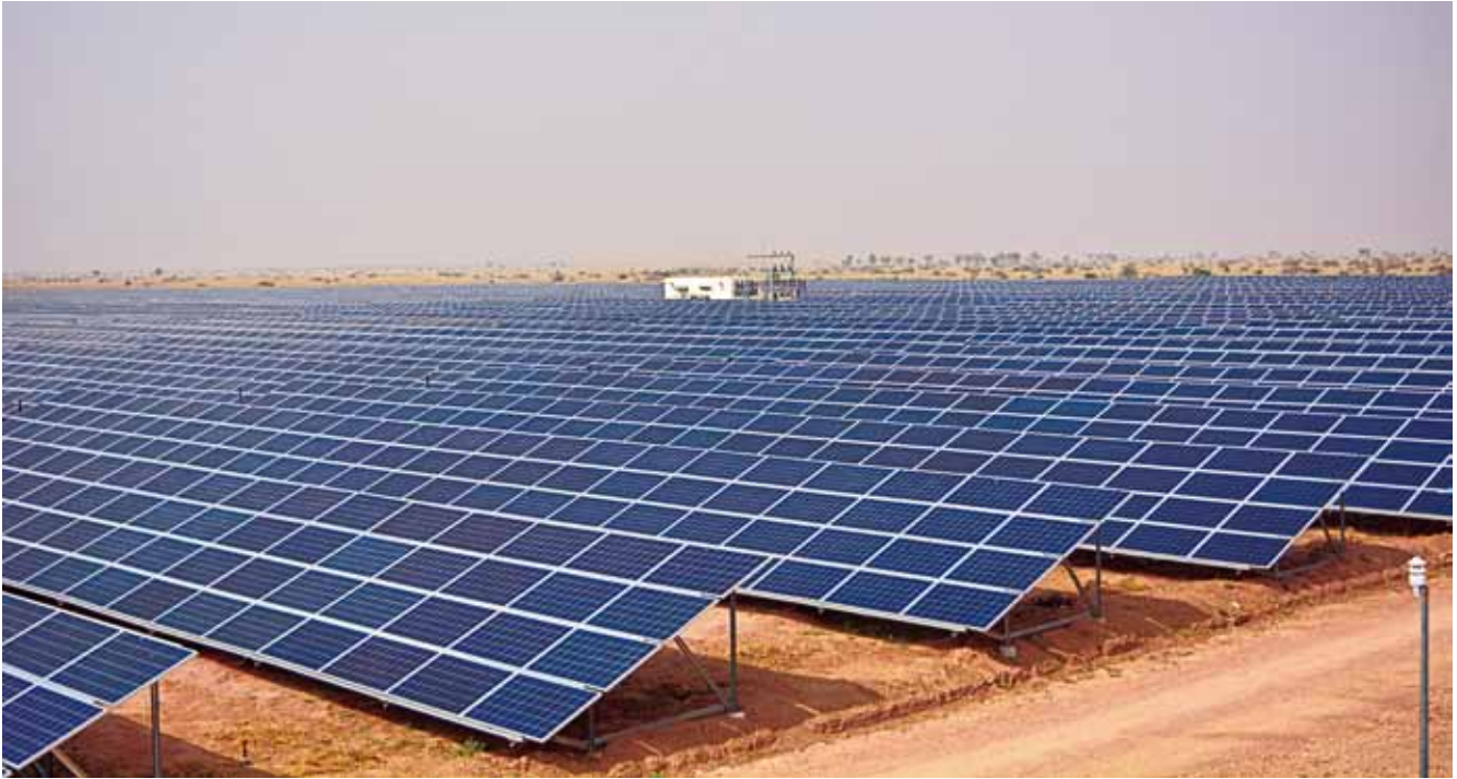
SECI 10 MW Project at Jodhpur, Rajasthan
