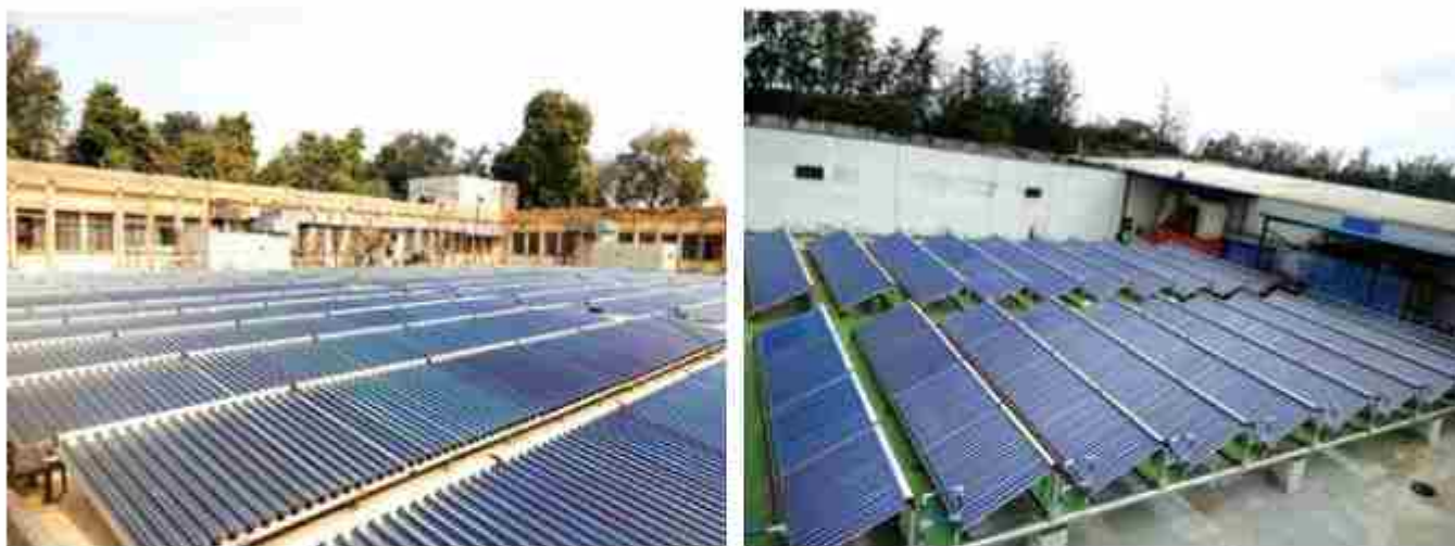
Fig. 3. CPC Collectors at GTPS, Gujarat and HUL, Amli
