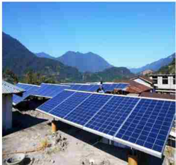
Solar Photovoltaic Power plant and Solar Water Heating Systems at District hospital in Arunachal Pradesh
