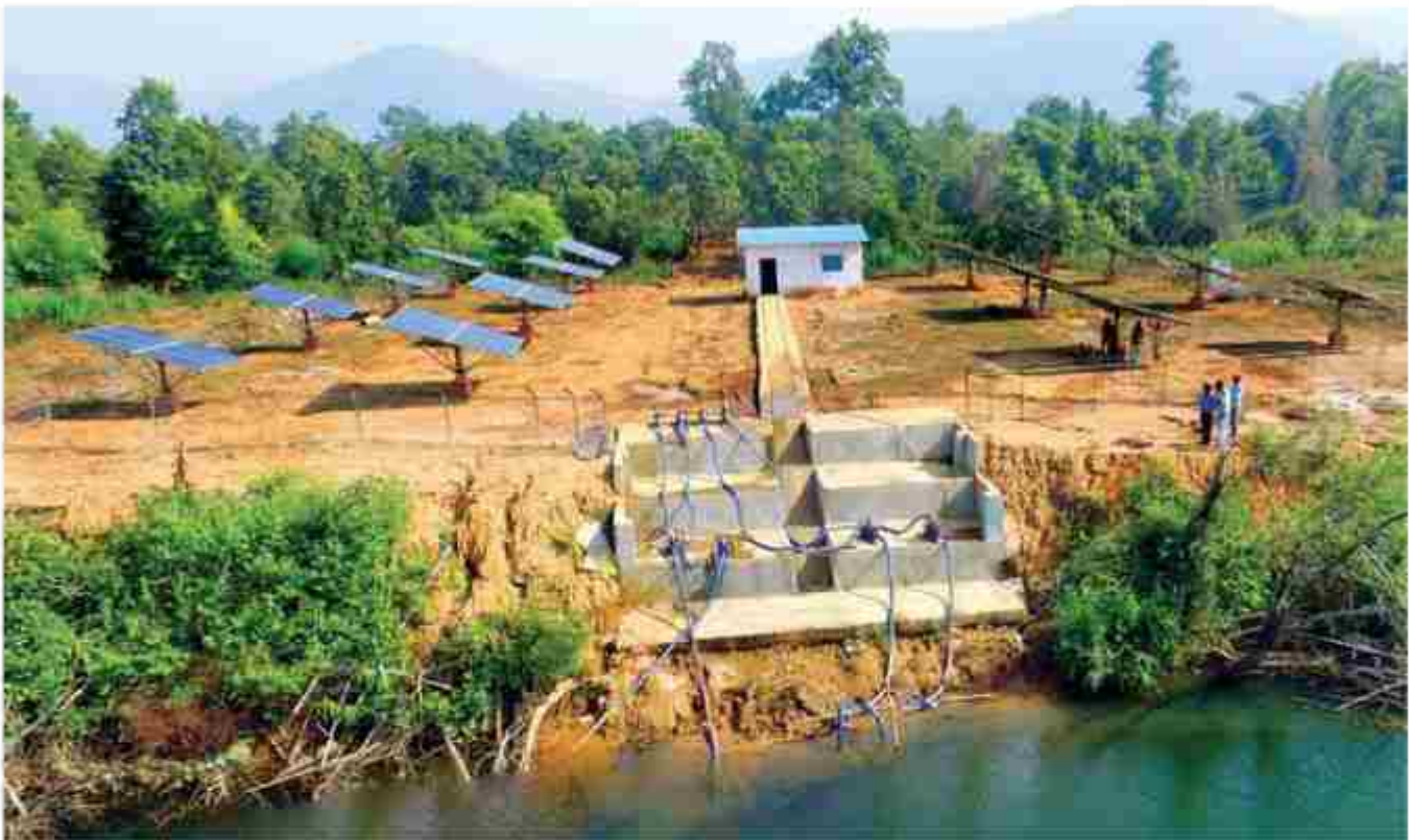
Community Solar Pump Systems installed at Kulhadiyhat Distt. Gariyabandh, Chhattisgarh
