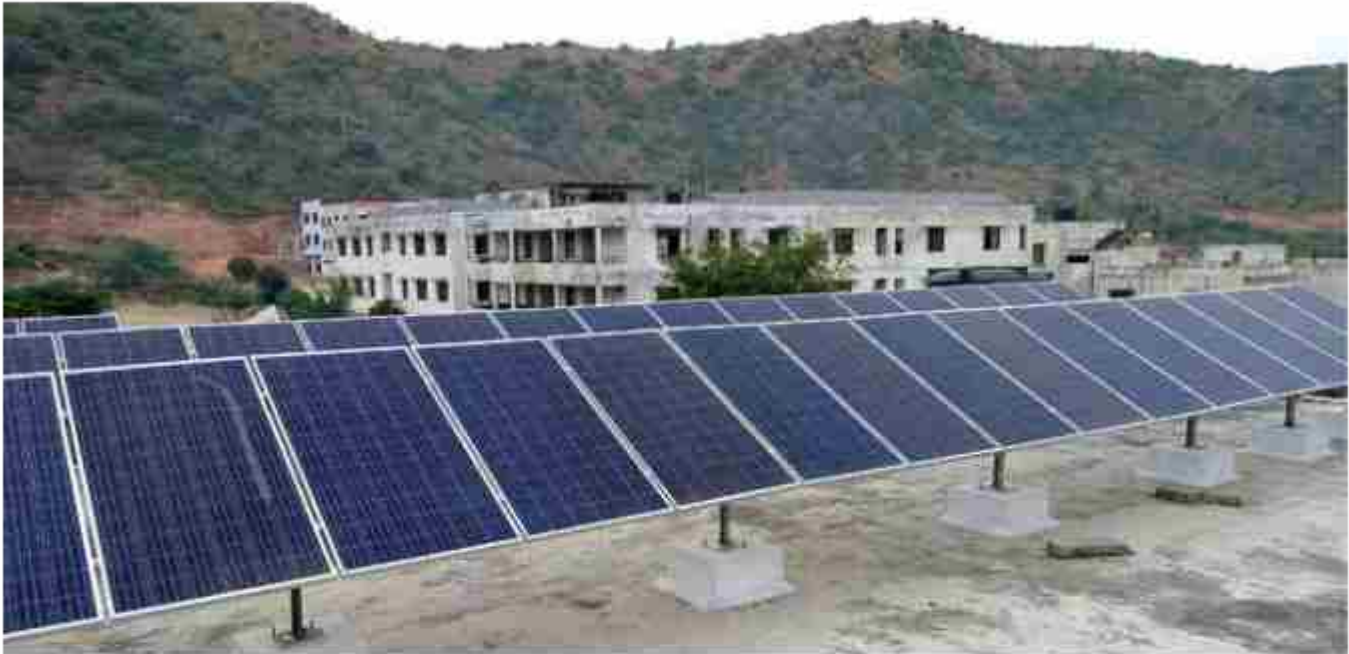
Grid connected solar rooftop plants of 300 kWp installed by SECI at SS College of Engineering, Udaipur, Rajasthan
