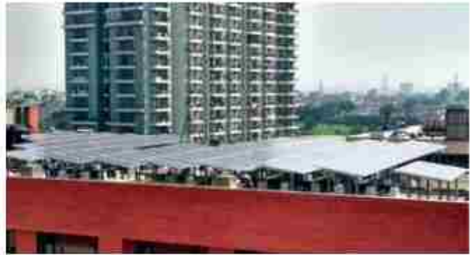
Grid connected solar rooftop plant of 170 kWp installed by SECI at Seth Anandram Jaisuria Education Society, Jaisuria Institute of Management, Indrapuram, Ghaziabad, Uttar Pradesh
