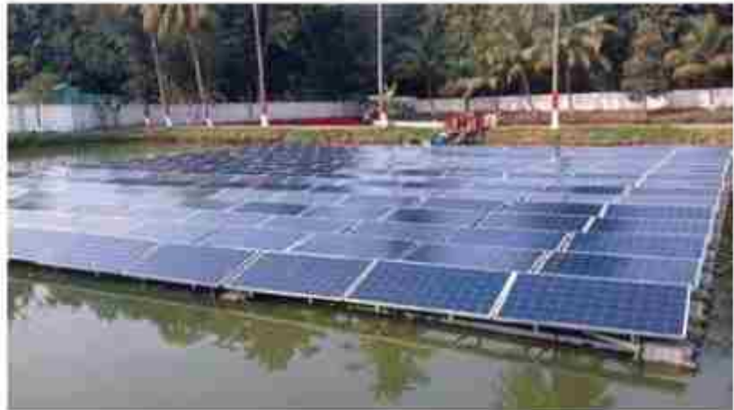
Installation of 60KWp Floating Pond Top Solar Power Plant at Hon'ble Governor House in Bihar
