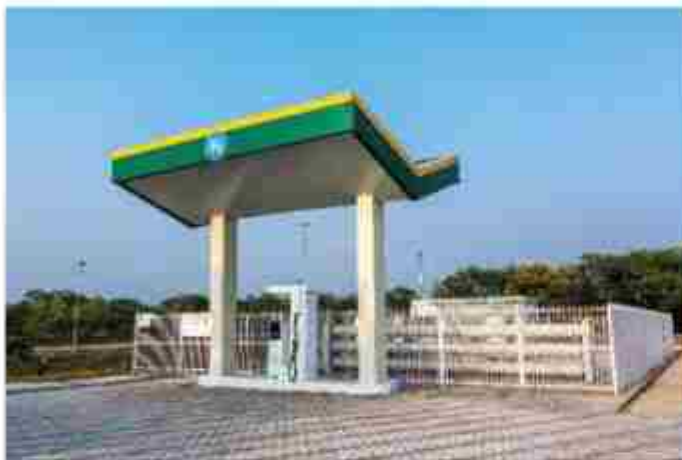
Hydrogen facility at NISE
