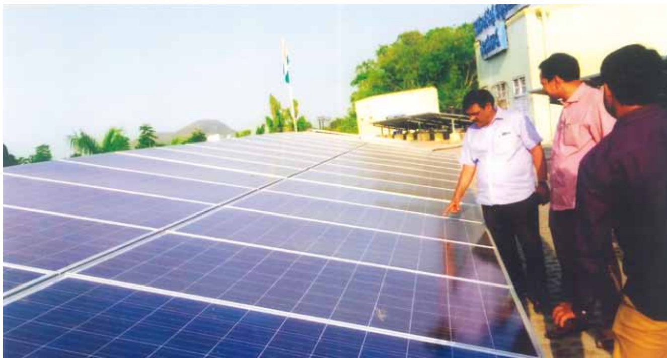
100 kWp Grid Connected Solar rooftop Power Plant at Municipal Office & Council Hall Building, Vijayawada, Andhra Pradesh
