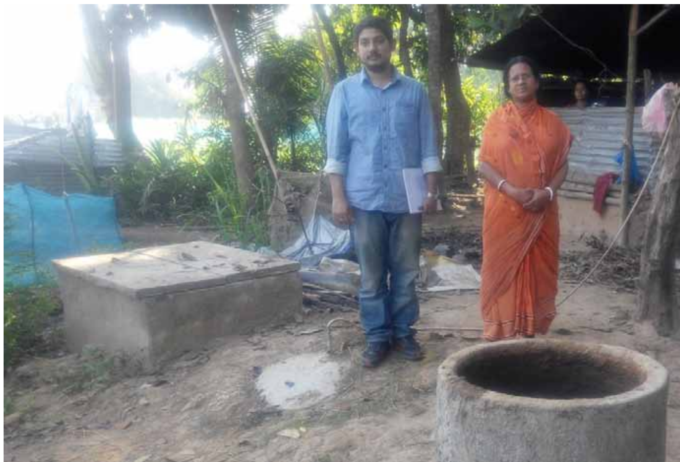
Deenabandhu Biogas Plant installed for beneficiary - Shri. Sudhir Das at village-Baidyamura, Nalchar RD Block, Tripura
