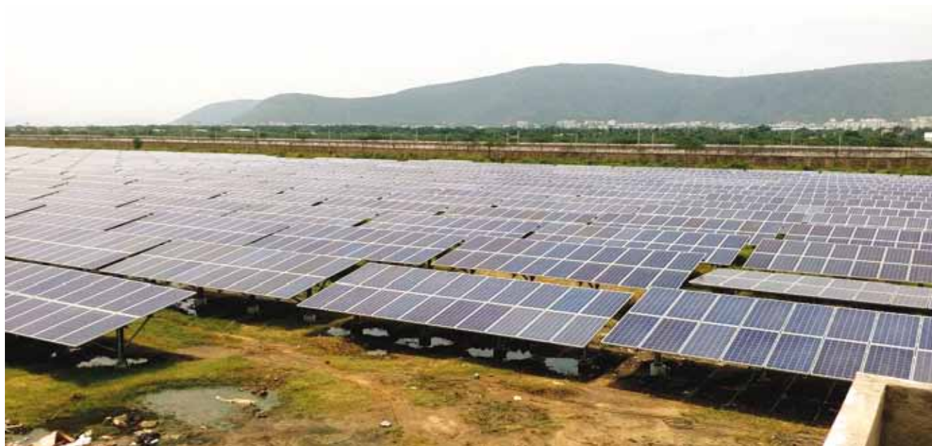
7.5 MW SPV Power Project at Vishakhapatnam Port Trust
