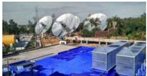
Installation of 570 sq. m of Paraboloid Dish at UltraMarine & Pigment Ltd., Tamil Nadu
