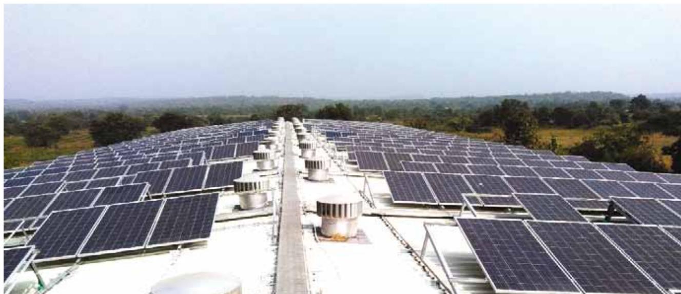
198 kWp grid connected solar rooftop plant at Pitambera Polymers Industries Pvt Ltd, Maharashtra
