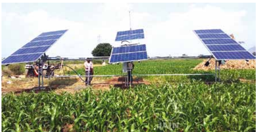
A 3 HP Solar Water Pump set-up at Kanpur Dehat, Uttar Pradesh
