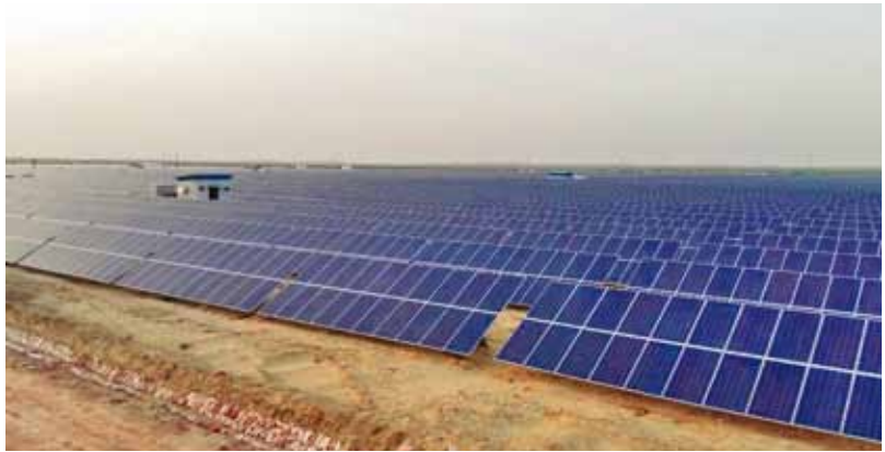
25 MW Solar Park at Solar Power Plant, Bhadla Phase-I
