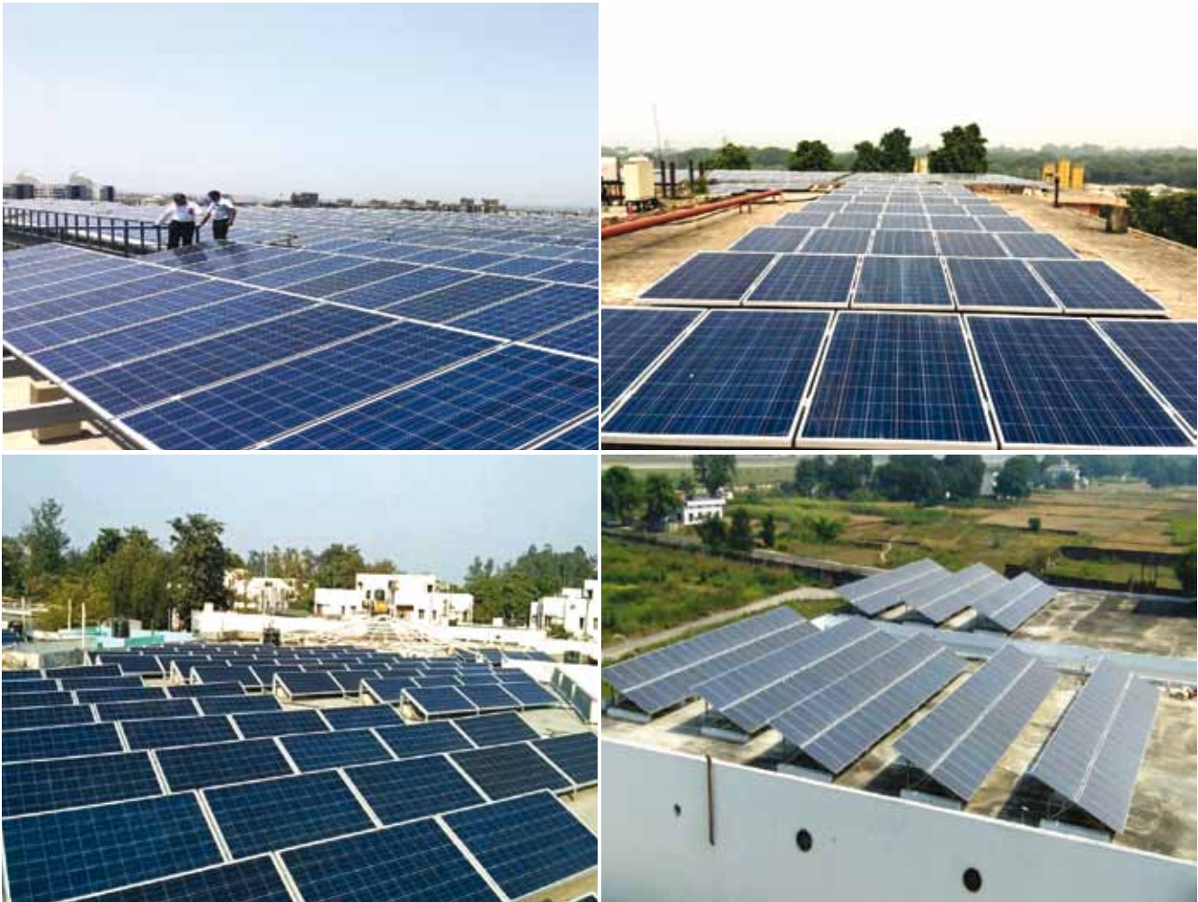
Projects commissioned under Grid connected Rooftop Schemes
