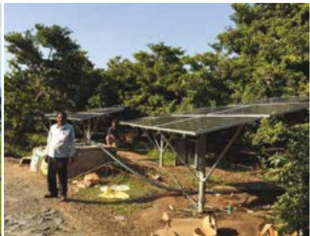
A Solar Pump at Dhundi village in Anand district, Gujarat
