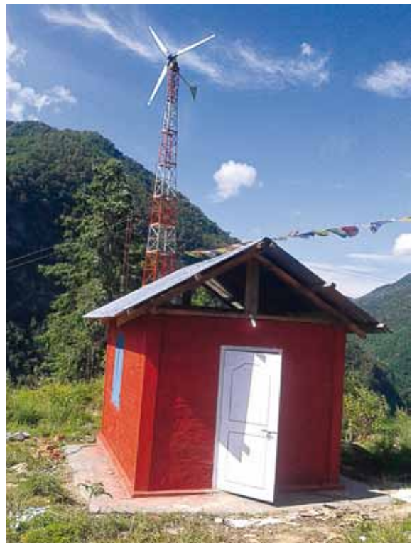
6.8 KW Wind-Solar Hybrid System in West Kameng, Arunachal Pradesh
