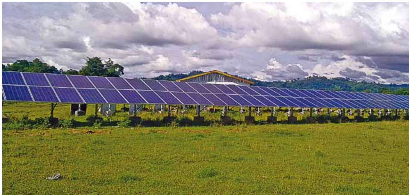
100 kW Solar Power Plant at Diyun
