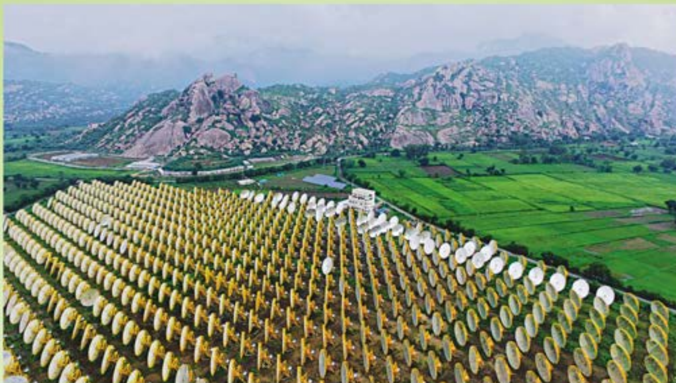
1.0 MW Solar Thermal Power Plant with 16 hr. Thermal Storage in Brahmkumari Ashram, Mount Abu
