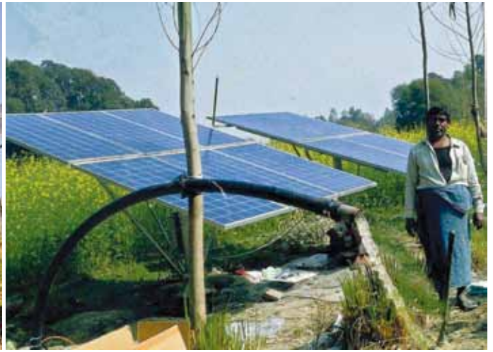
A 3 HP Solar Water Pump at Village Vasudevpur, Distt. Amethi, UP
