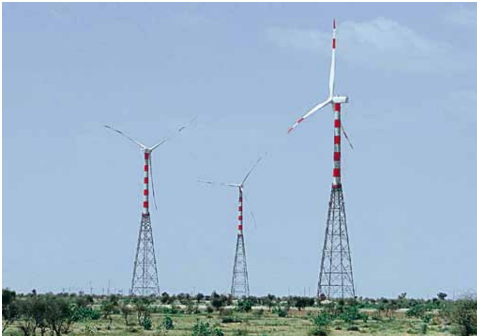
50.4 MW hybrid tower wind farm in Rajasthan
