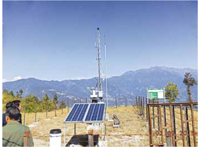
SRRRA Station at Gangtok, Sikkim
