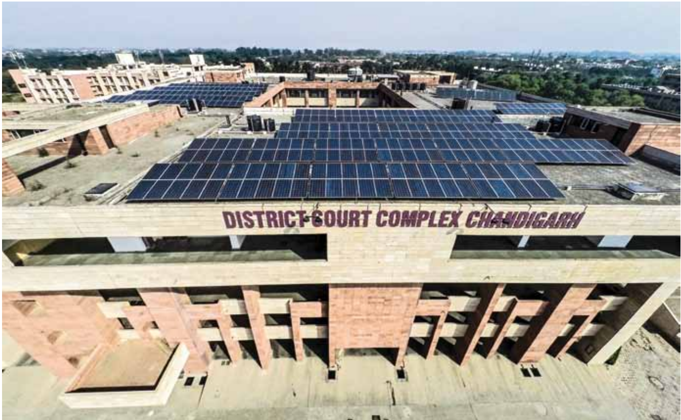
100 kW p grid connected solar rooftop power plant established at District Court Complex, Chandigarh
