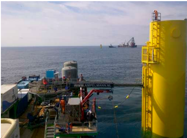
Figure 75 - Grouting spread on the aft of an offshore supply vessel - Borkum West II
