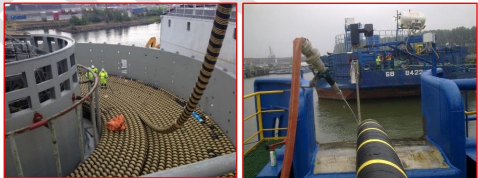
Figure 15 Right: Loading of cable into CLV turntable. Left: Transfer of cable from quayside chute to CLV chute.
