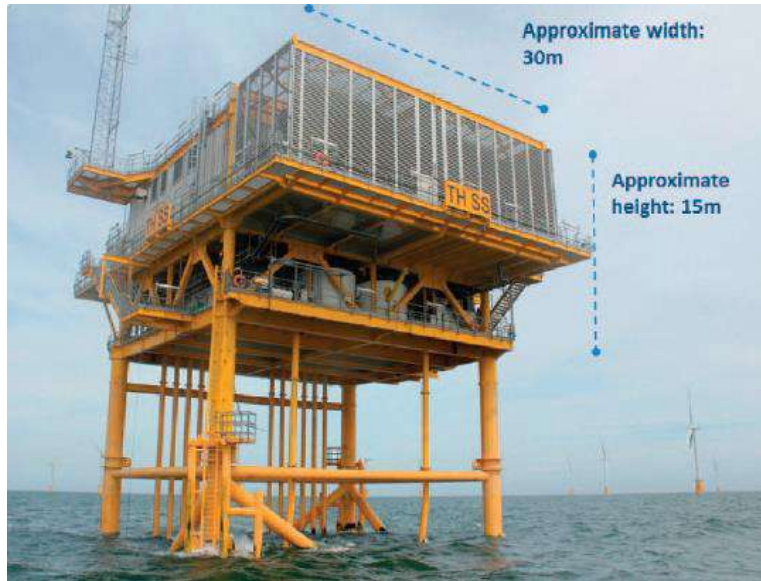
Figure 29: An example of an offshore HVAC Substation [31]
