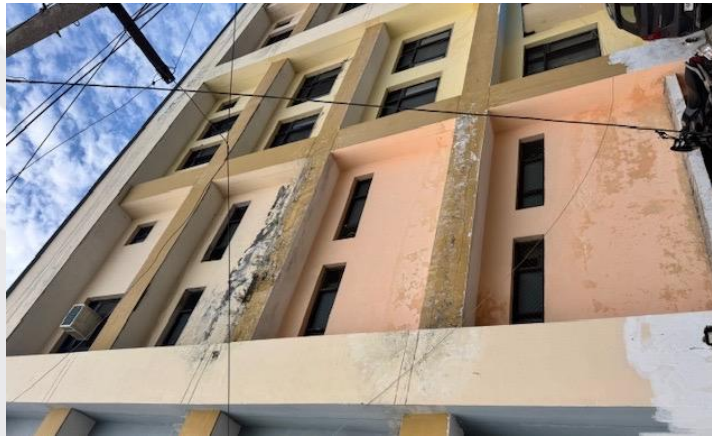
Fig. 2 WC LEAKAGE DAMAGING OUTERSIDE OF BUILDING
