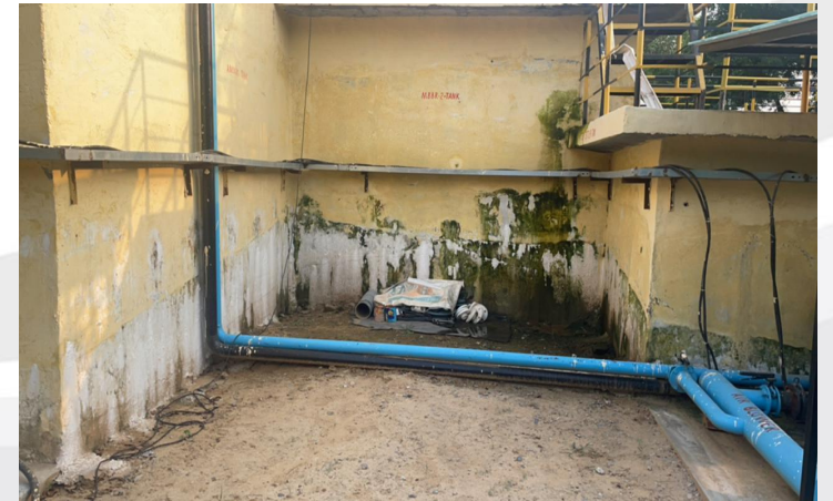
Fig. 3 STP PLANT CONCRETE FAULTS
