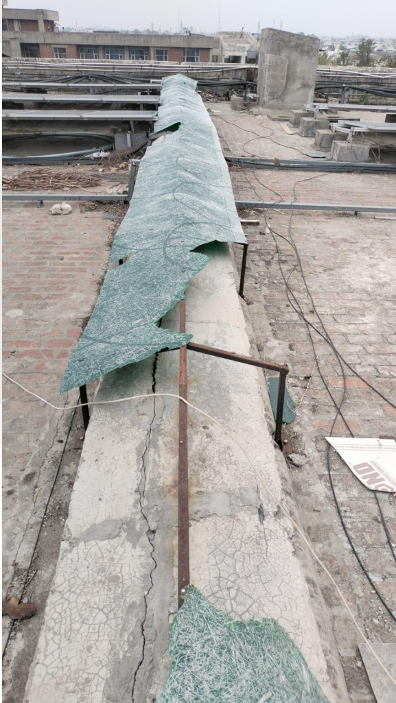
Expansion Joint Breakage
