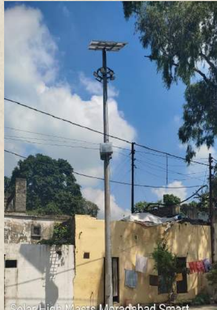
Solar High Masts Moradabad Smart City Shaffer Energy Pvt Ltd 20.09.2021 11:03 28.84386, 78.76507 Pili Kothi, Near Cross Road Mall, Civil Lines, Moradabad, Uttar Pradesh 244001 Company Bagh
