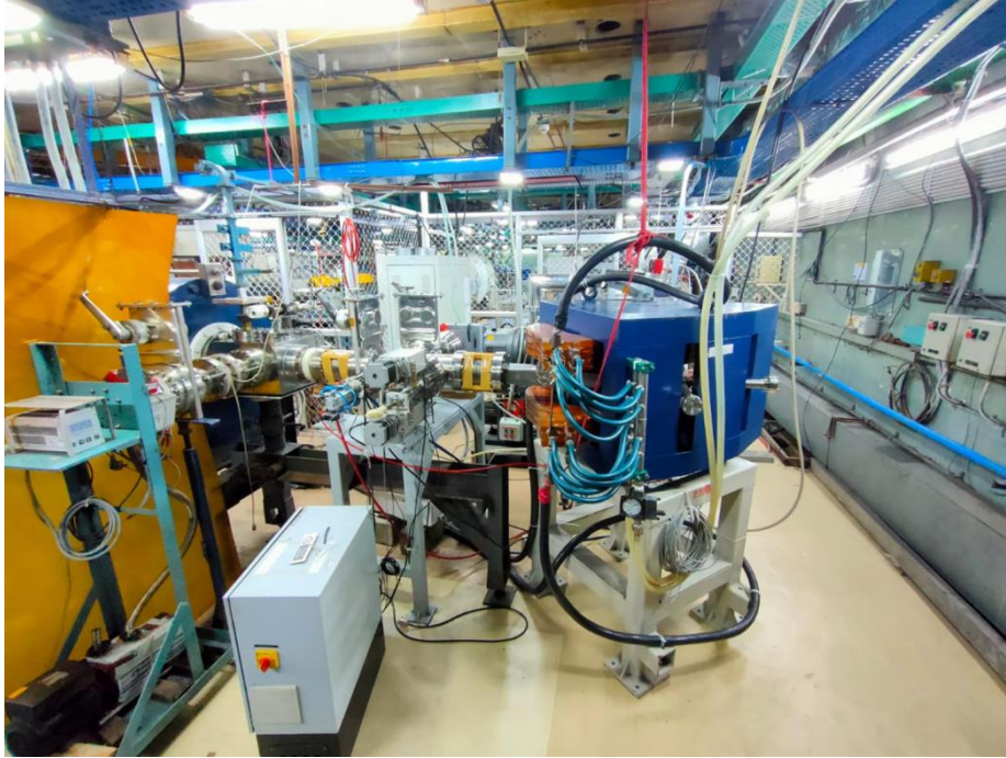
Fig. 4.1.6: RIB facility installed in one of the experimental caves of the K130 Cyclotron
