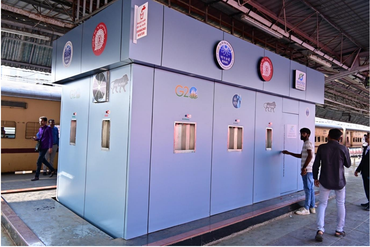
Picture of 750 LPH capacity water purification unit installed at PF-14/15, CSMT, Mumbai
