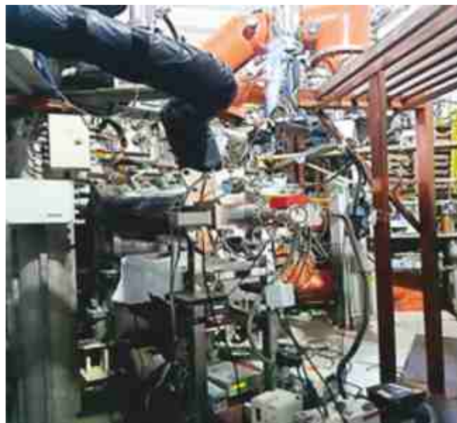
View of installed sorption pump on the radial port of the SST-1 Tokamak
