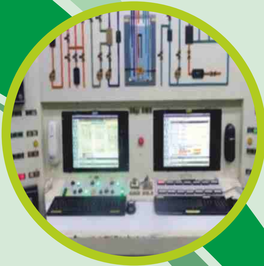
Operator Console of ICIS of KAMINI Reactor
