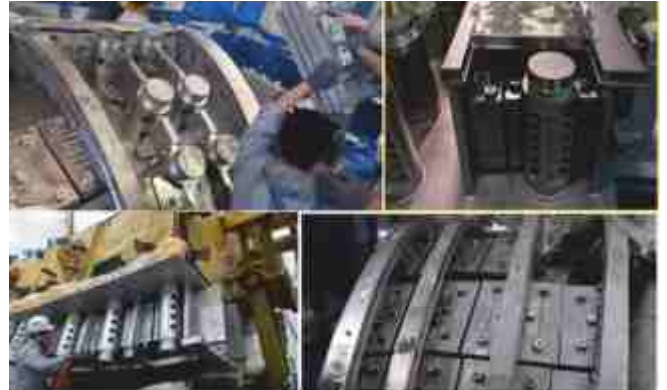
In sequence: IWS lowered for assembly in VV sector, IWS assemble around flexible support housing between outer and inner shells of VV, inspection after assembly to ascertain needed clearance, VV segment view after assembly of IWS and ready for welding the outer shell
