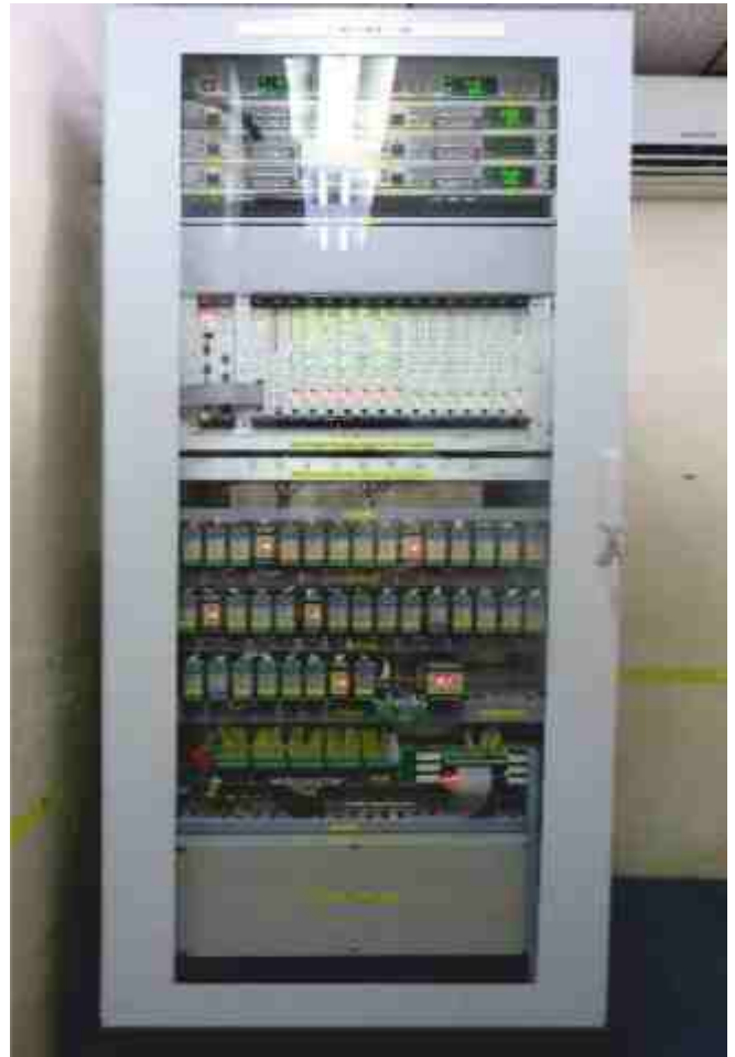
Sub-System-II Panel of ICIS of KAMINI Reactor
