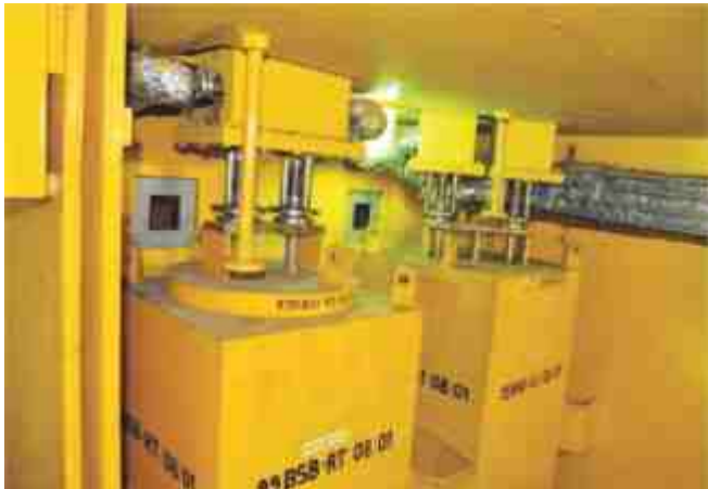
Ion Exchange columns at PHIX System for treating of legacy Intermediate Level Liquid Waste
