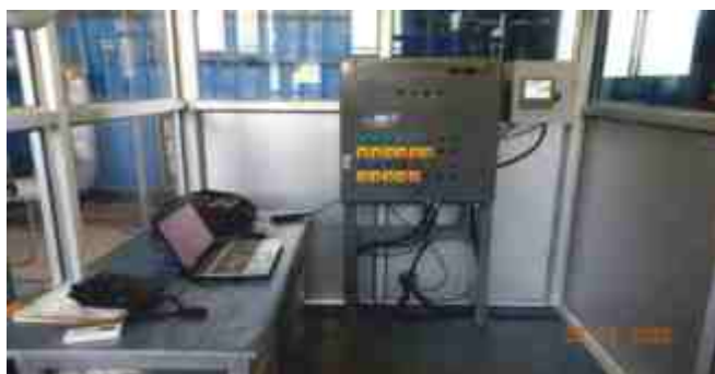
New LOCA Chamber Control Room
