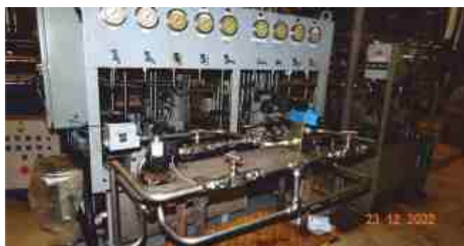
Proportional Flow Control Valves Testing in FMTF
