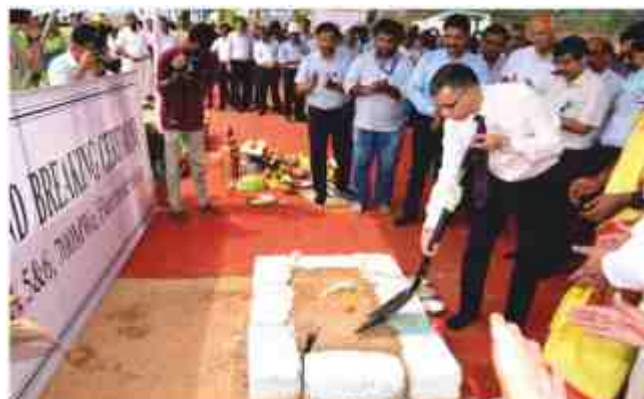
Excavation at Kaiga Project Unit-5&6 Main plant commenced with ground breaking on April 28, 2022
