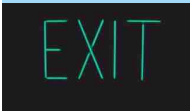
GTLS 'EXIT' sign board under dark
