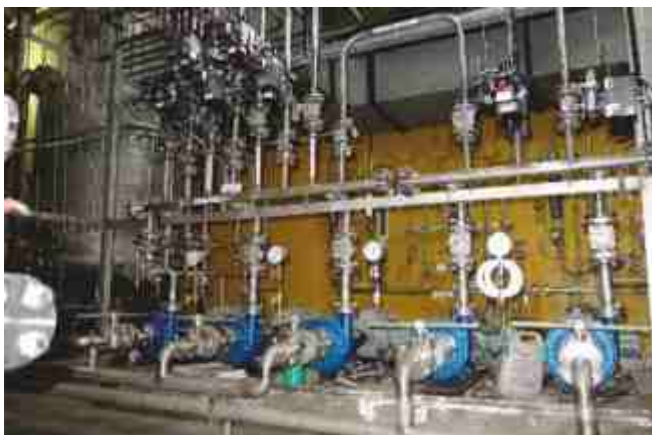
Effluent Conditioning and Transfer System for processing of MWPF laden waste
