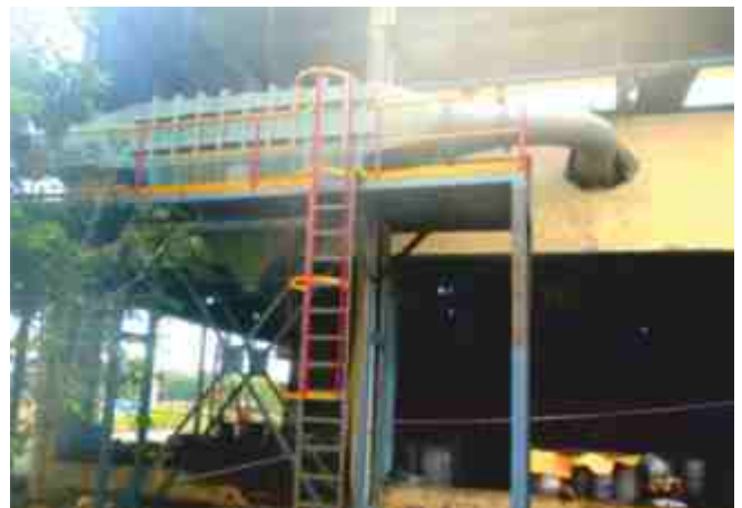
Solid Trap at Chlorination Section
