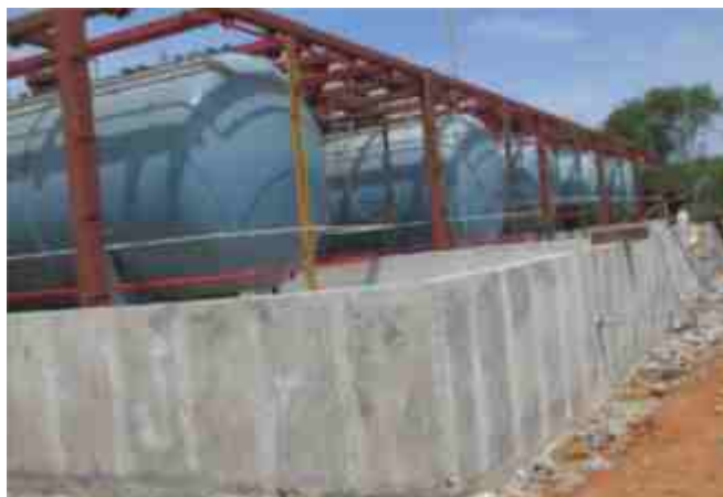
Storage tanks installed at SPP with MVWS system, HWP, Tuticorin
