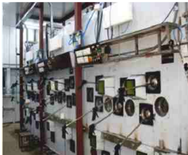
I-131 processing facility at CIRUS
