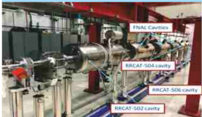
String Assembly for pCM of PIP-II with 3 cavities from RRCAT, India and 3 from Fermi lab, USA
