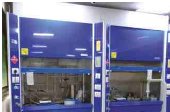
The fully refurbished laboratory facilities of Effluent Treatment Plant in Trombay
