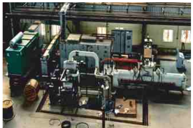
Plasma Melting furnace – commissioned
