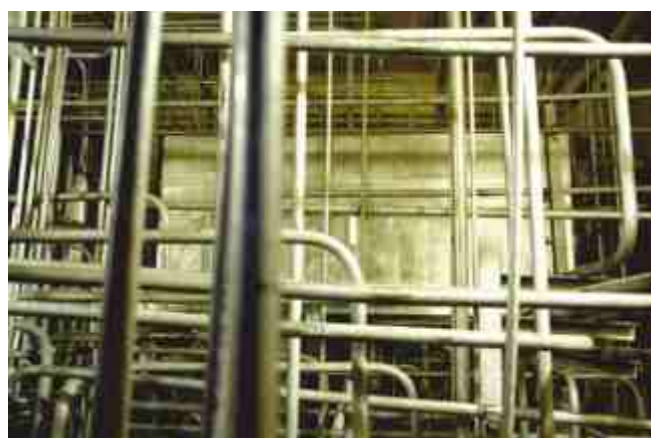
The In-cell Mixer Settler Unit of Waste Immobilisation Plant in Trombay
