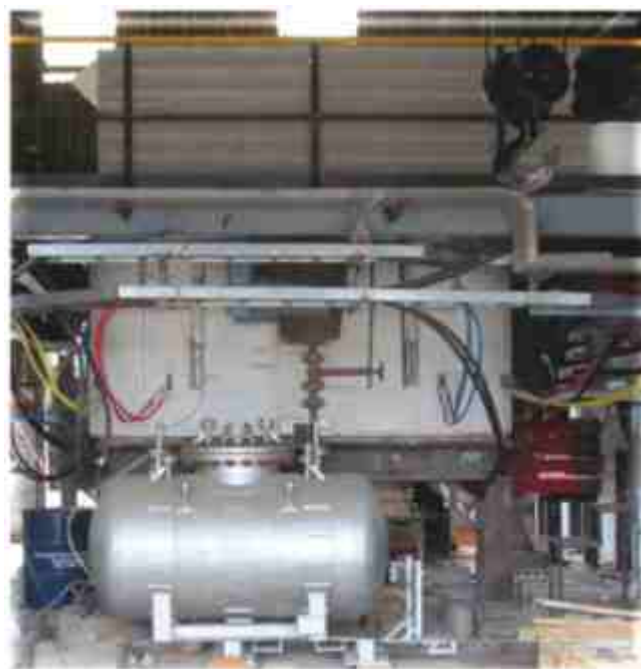
24 kA Cell at HWBF, Vadodara
