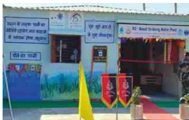
The 12500 litres per hour capacity water treatment unit based on BARC technology commissioned at BSF outpost at Kutch near Indo-Pak border
