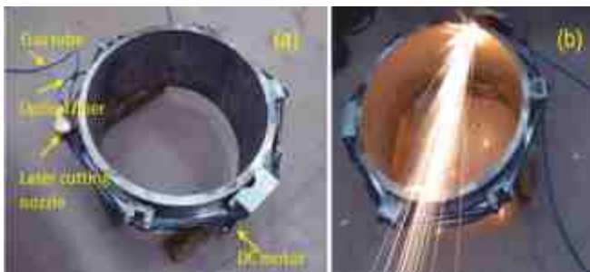
Laser cutting tool and mock trial of 30 mm thick and ~700 mm dia. SS316L tube for cutting of recirculation loop at TAPS-1&2 using 1 kW average power Nd: YAG laser
