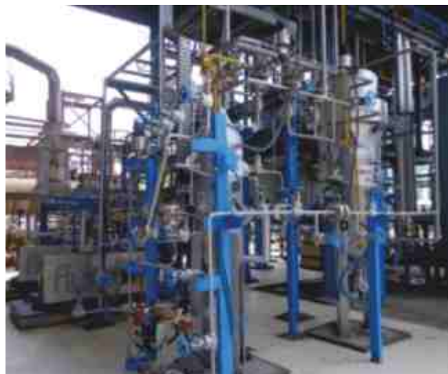
Boron Trifluoride production facility at HWBF, Talcher
