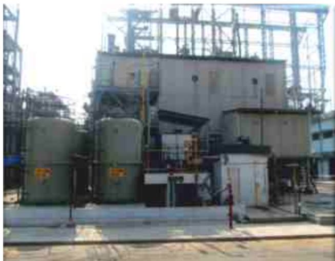
Scrubber system for 24kA sodium cell at HWBF, Vadodara
