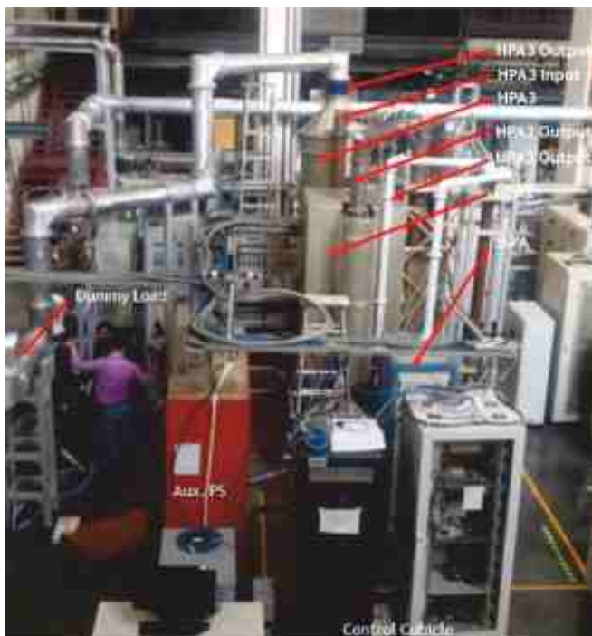
View of Installed RF source in SST-1 hall
