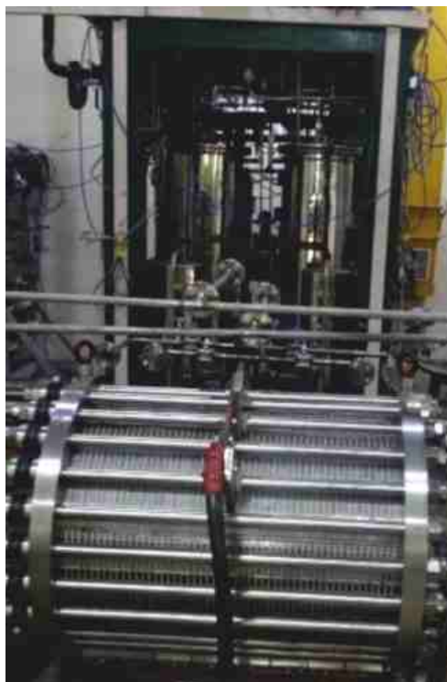
Alkaline Water Electrolyzer plant integrated with a 50 cell stack
