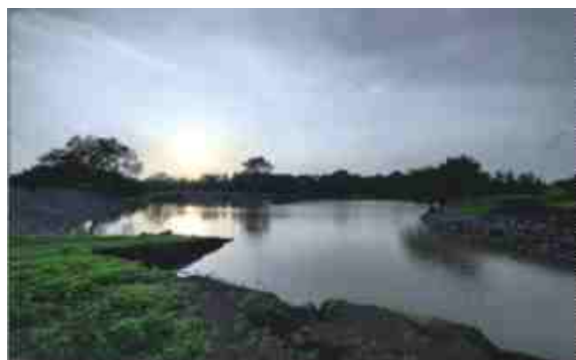
Check dam at Indu village, Tapi District, Gujarat
