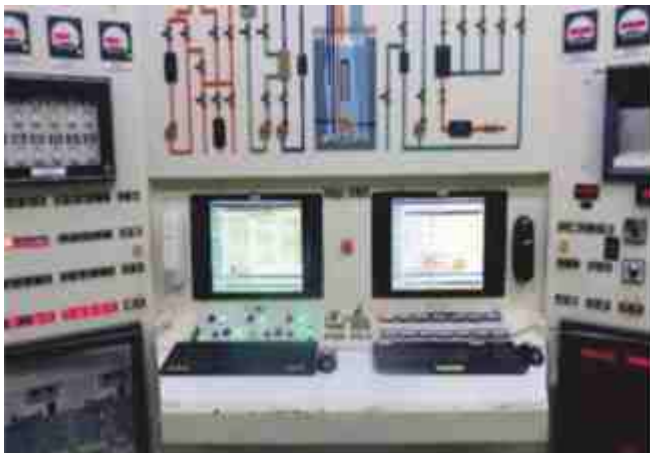
Operator Console of ICIS of KAMINI Reactor
