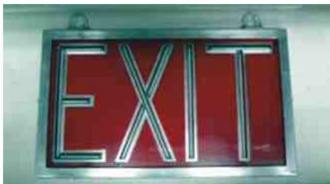
GTLS 'EXIT' sign board in day light
