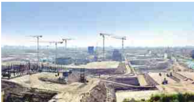
Main plant area of GHAVP-1&2
