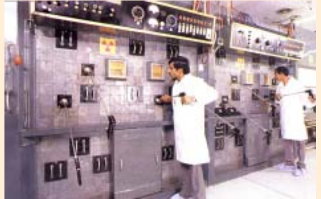
Hot-Cells : Radioisotope production facility at BARC
