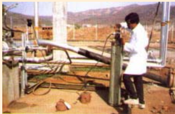
Leakage in pipe being detected with the help of radiotracer
