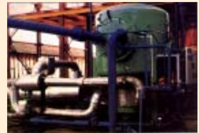
Low Temperature Evaporation Desalination Plant (Capacity : 30 cubic metre per day)
