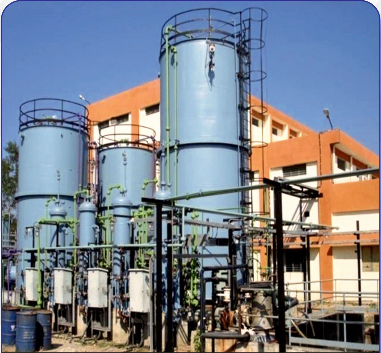
Boron Enrichment Plant at Heavy Water Plant, Manuguru
