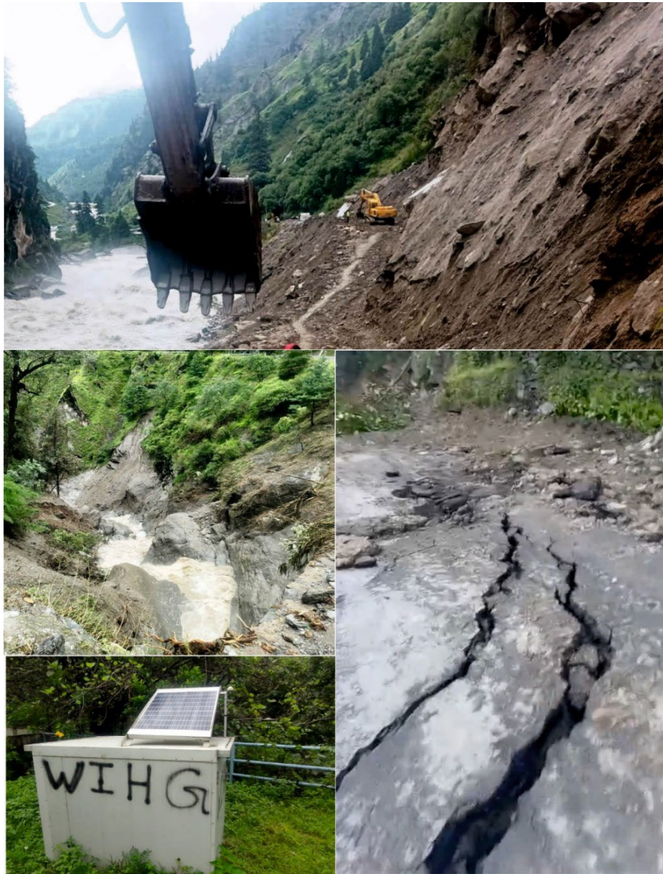
Figure 4. Showing the road condition along the Gangotri Highway, where debris flows have washed away sections of the road, caused cracks, and rendered the flood-affected Bhagirathi valley without any motorable route.
