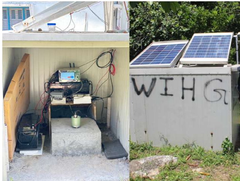
Figure 5. Photograph of the IGM integrated with the BBS at the Maneri site, showing the complete field installation. The system is powered by two solar panels and supported by two batteries, providing a reliable and continuous power supply for uninterrupted operation under field conditions.
