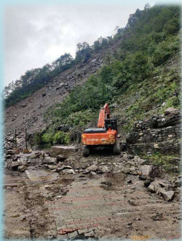
Entire road washout due to landslide
