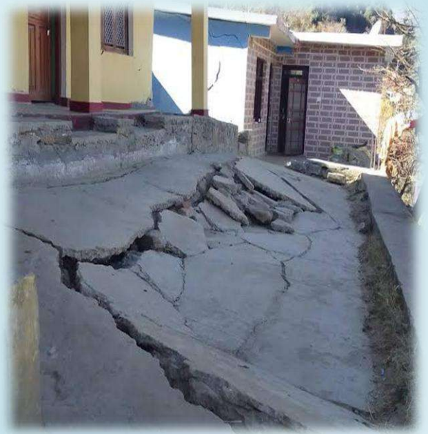
Cracks and Subsidence of ground
