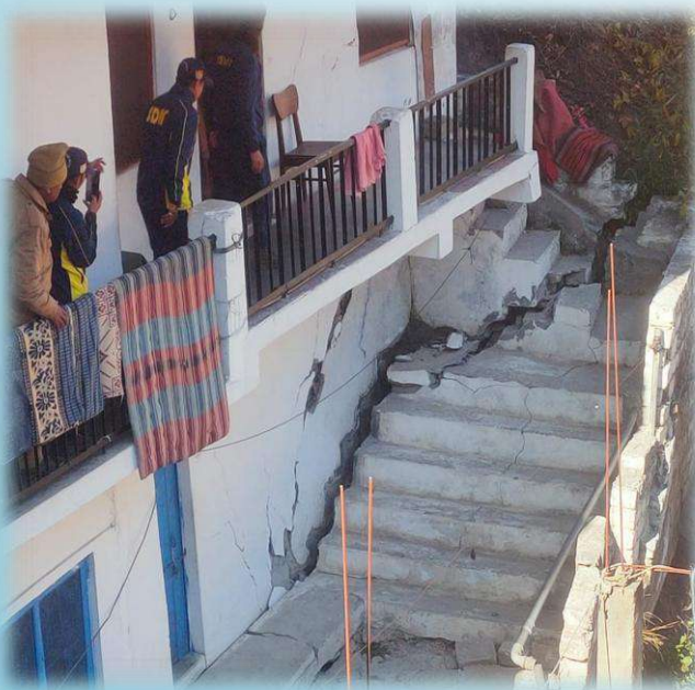
Cracks on walls due to ground
