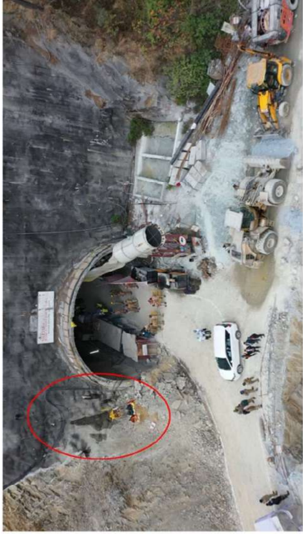
In Figure 18, the site is portrayed with a red-coloured circle highlighting a subtle water seepage from the ground. This minor concern was addressed promptly at that specific moment.
