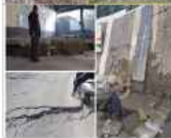
Fig. 9. The frames and ground deformations observed adjacent to the bridge region at 23 miles.
