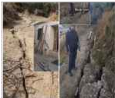
Fig. 3. Structural damage of Muzum high rise in the basement forming with extensive damages to the structure
