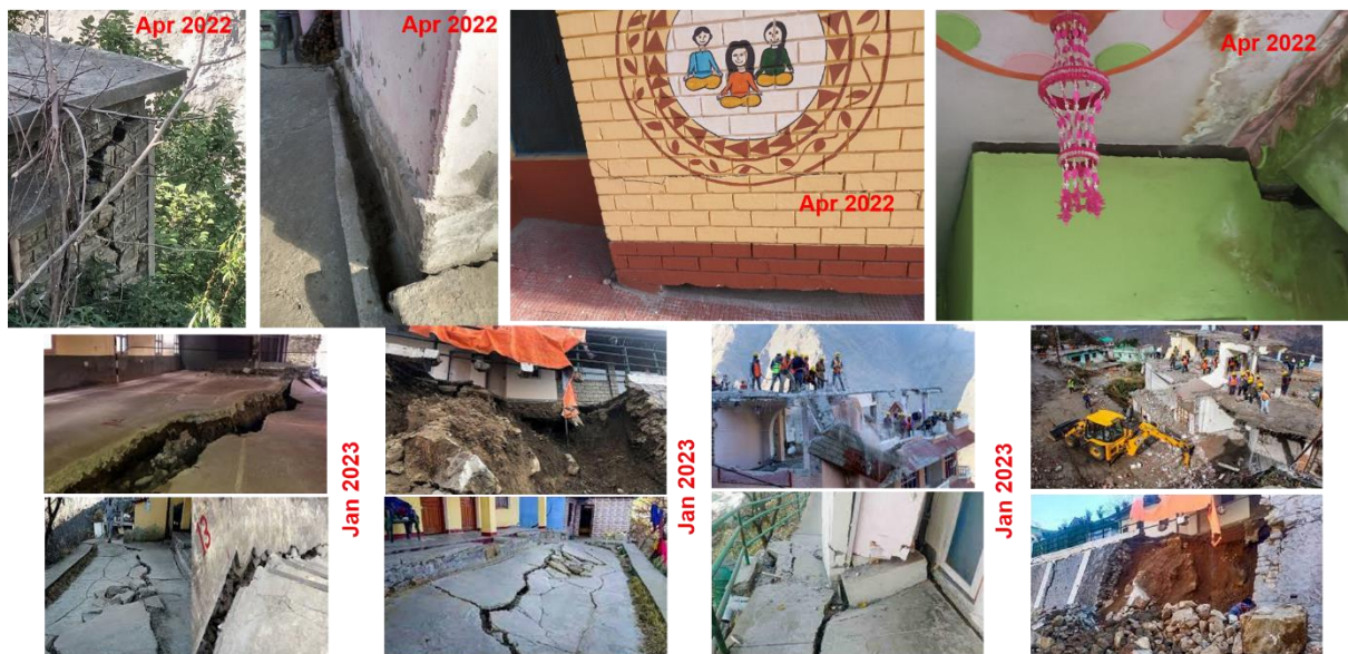
Figure 6: Field information of the damage to infrastructure and houses due to land slippage in Joshimath Town collected during field visit in April 2022 and collected from social media in January 2023
