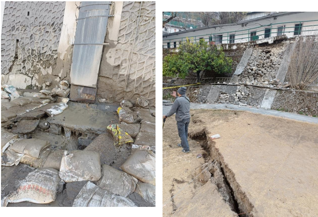
Fig. P10: Damage to retaining wall and play-ground at Marwadi (MW) near Jaypee Colony
