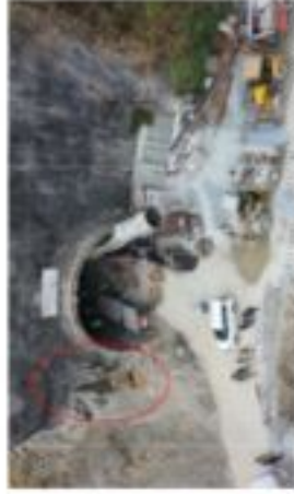
In Figure 18, the sub is positioned with a red colored circle highlighting a white water escape from the ground, this water coming was addressed promptly at that specific moment.
