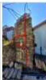
Photo 2.12: Possible line of discontinuity due to a crack at Nanyang temple
