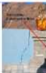
Photo 5.10 Opening of Construction joint along two different segments of wall.
