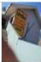
Photo 5.9 Opening of Construction joint along two different segments of walls.
