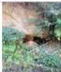
Photo 4.14 Removal of tree roots resulting in the flow below the giant tree
