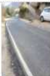
Photo 6.7 Crack in the thick top layer of Road near Yotat Givat
