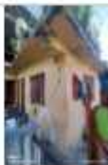
Photo 4.3: CMV Crack in the house near the Subari house at Nandipati.
