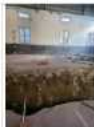
Photo 4-1 Vertical Ground Crack at JP Colony (Marine)
