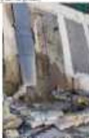
Photo 1.6 Destroyed Spring outlet at the gate of St. Tikhon's Masole
