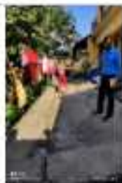
Photo 4.2: Fld Crack on the floor of the house of Mr. Subari at Nandipati.
