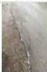
Photo 6.8 Crack in the thick top layer of Road in Sdeh area
