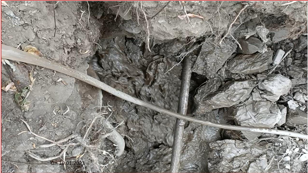
Fig. 1: Photograph of the site of gushing water at Jaypee Colony (Date: 08.01.2023)
