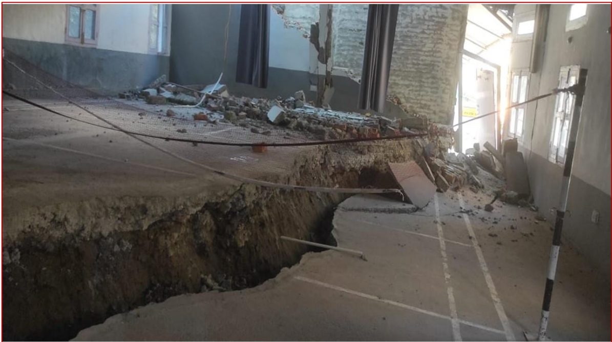
Fig. 2: Photograph of land subsidence very close to the gushing water site in the Badminton court of Jaypee Colony
